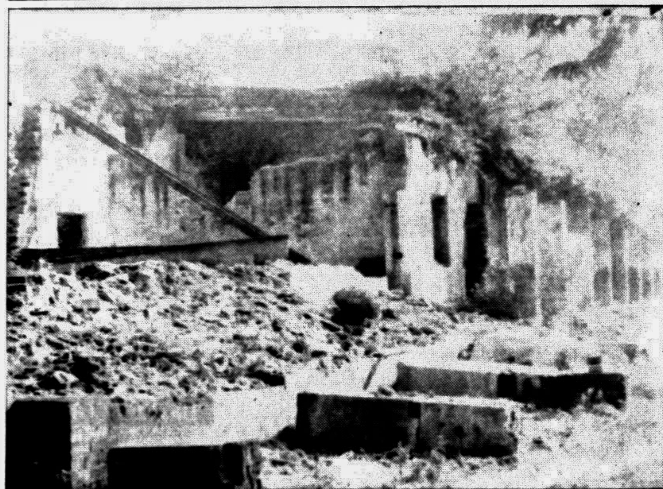
RANGPUR: A century old abandoned hostel building of Rangpur Zilla School poses as a threat to the school boys' lives who use to play nearby during their recess. The dilapidated building cannot be abolished due to fund shortage. — Star photo
