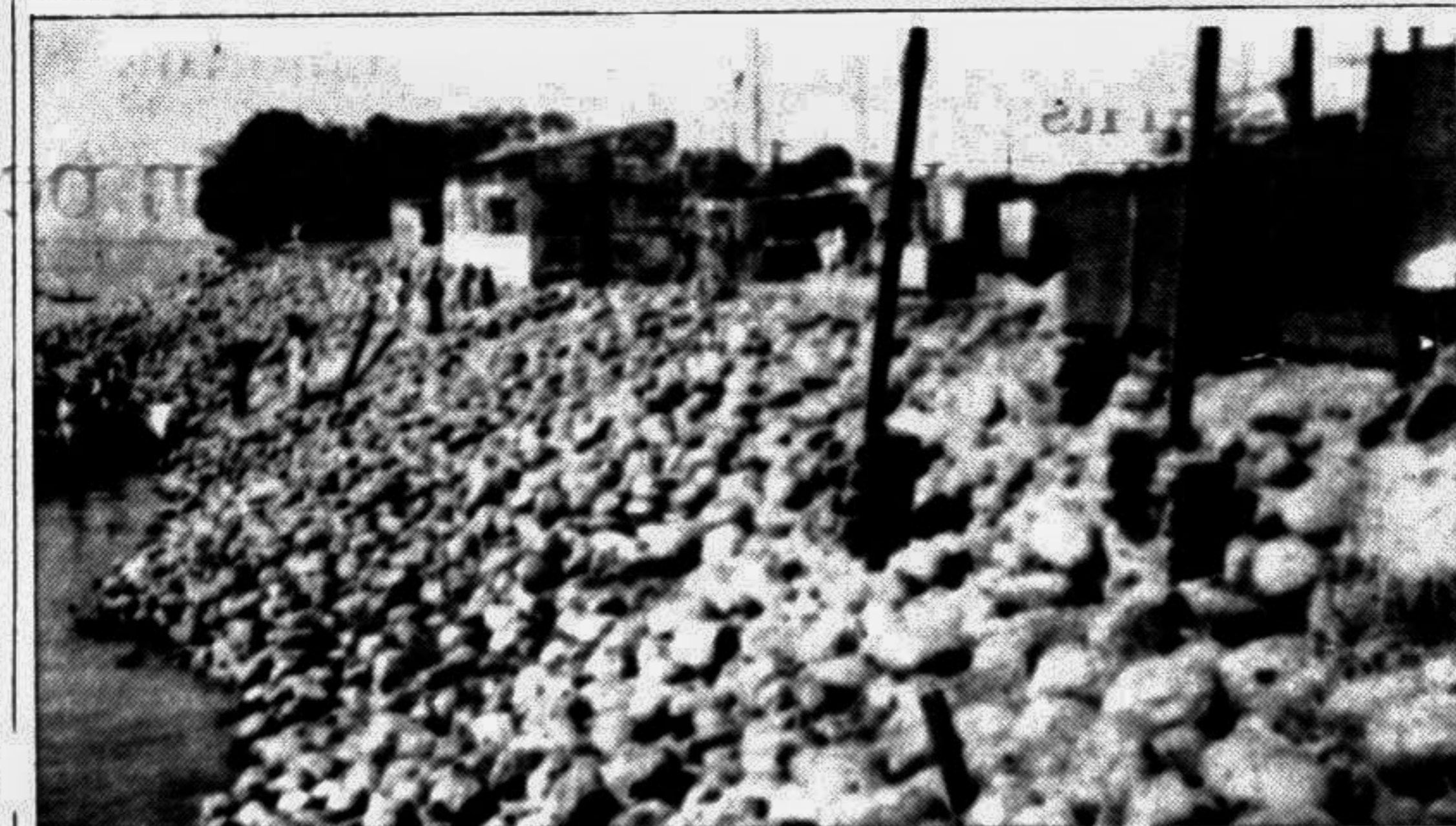
CHANDPUR: Huge boulders were placed along the bank of the river Meghna by Bangladesh Water Development Board to protect Chandpur town from erosion.— Star photo
