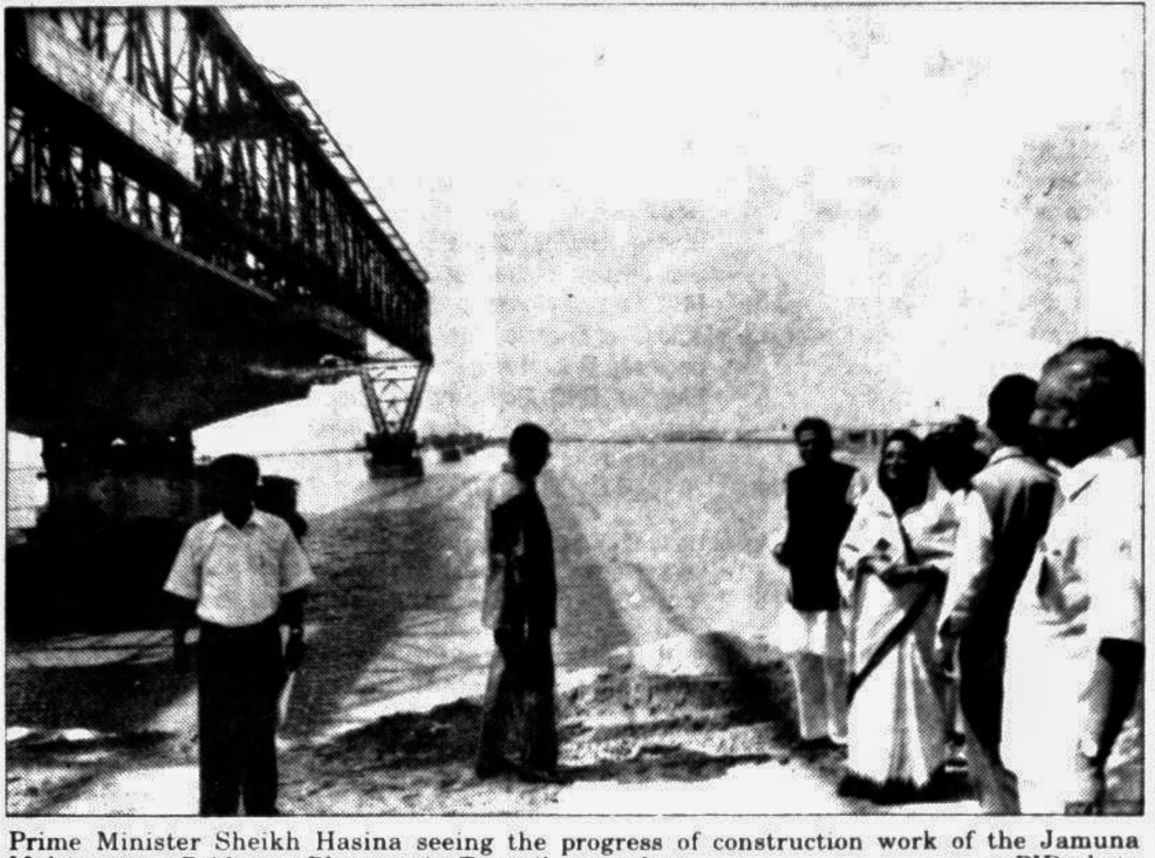
Prime Minister Sheikh Hasina seeing the progress of construction work of the Jamuna Multipurpose Bridge at Bhupur in Tangail yesterday. — PID photo
