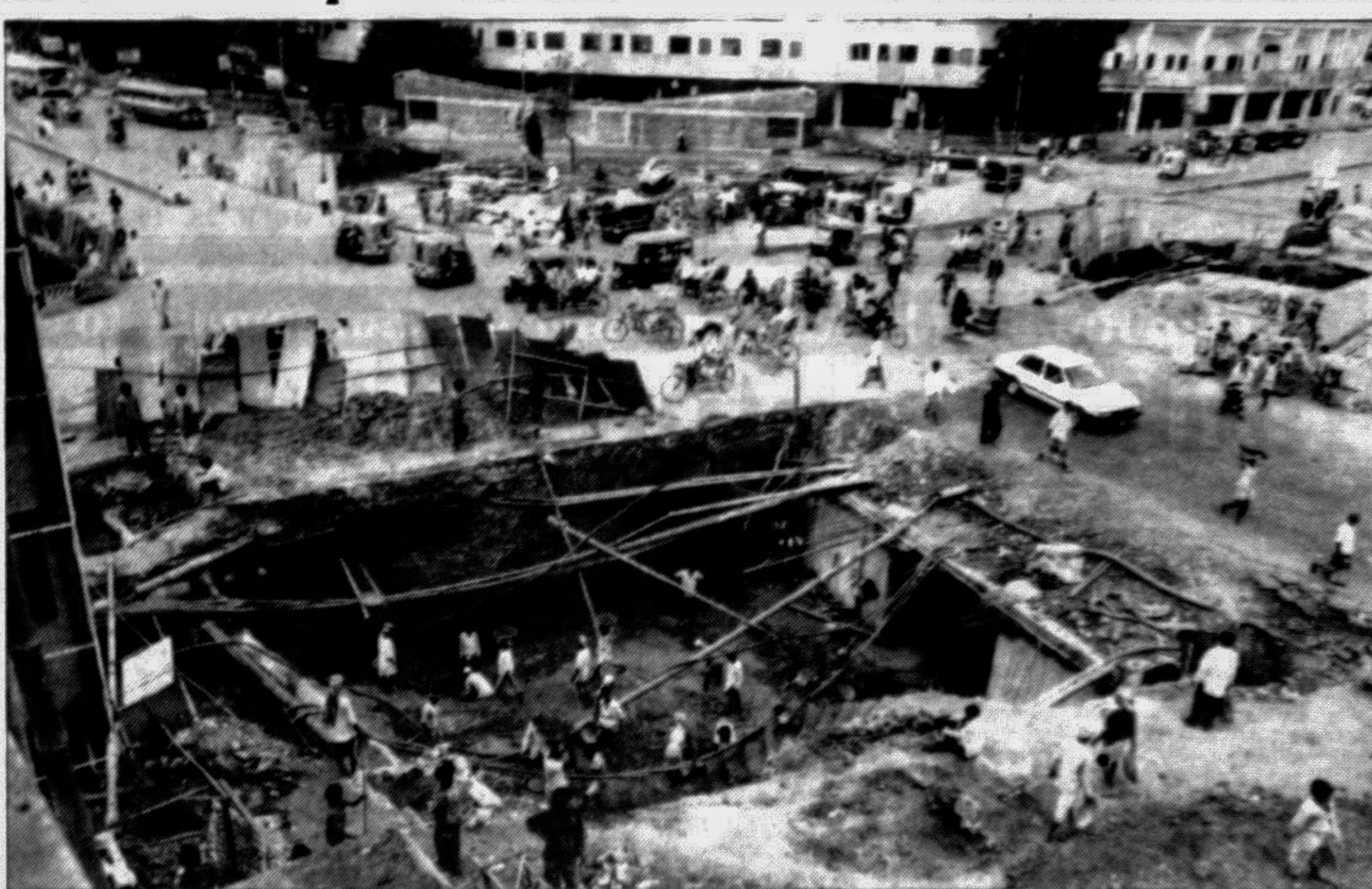
Construction work on an underpass going on at Gulistan in the city.
