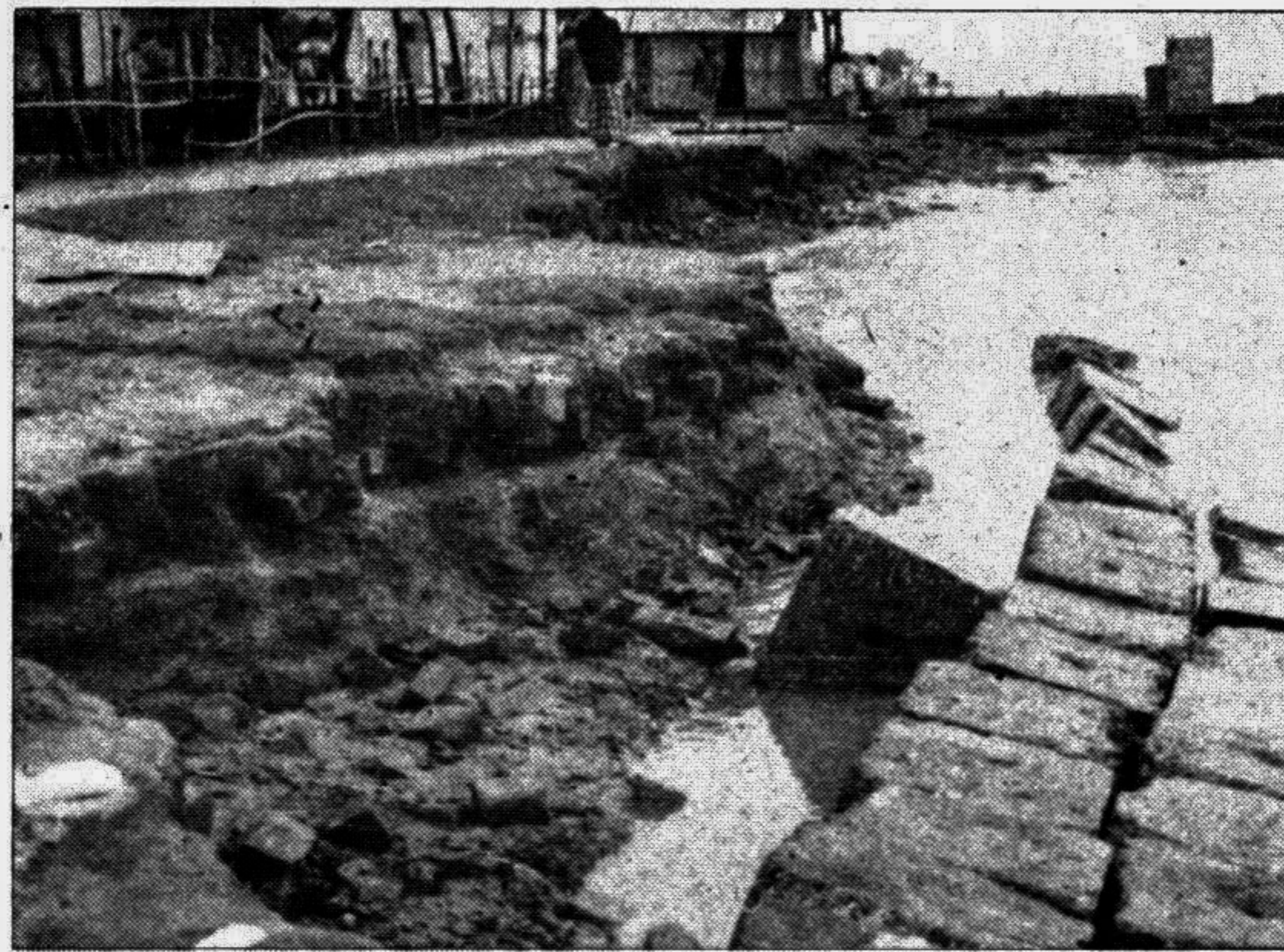
A FRUITLESS EFFORT: The picture showing a portion of bank of river Meghna in Natunbazar area where the Bangladesh Water Development Board authority made an effort to check further river erosion in the Chandpur town area recently. Most of the concrete blocks were, however, washed away and the rest may vanish any day. — Star photo
