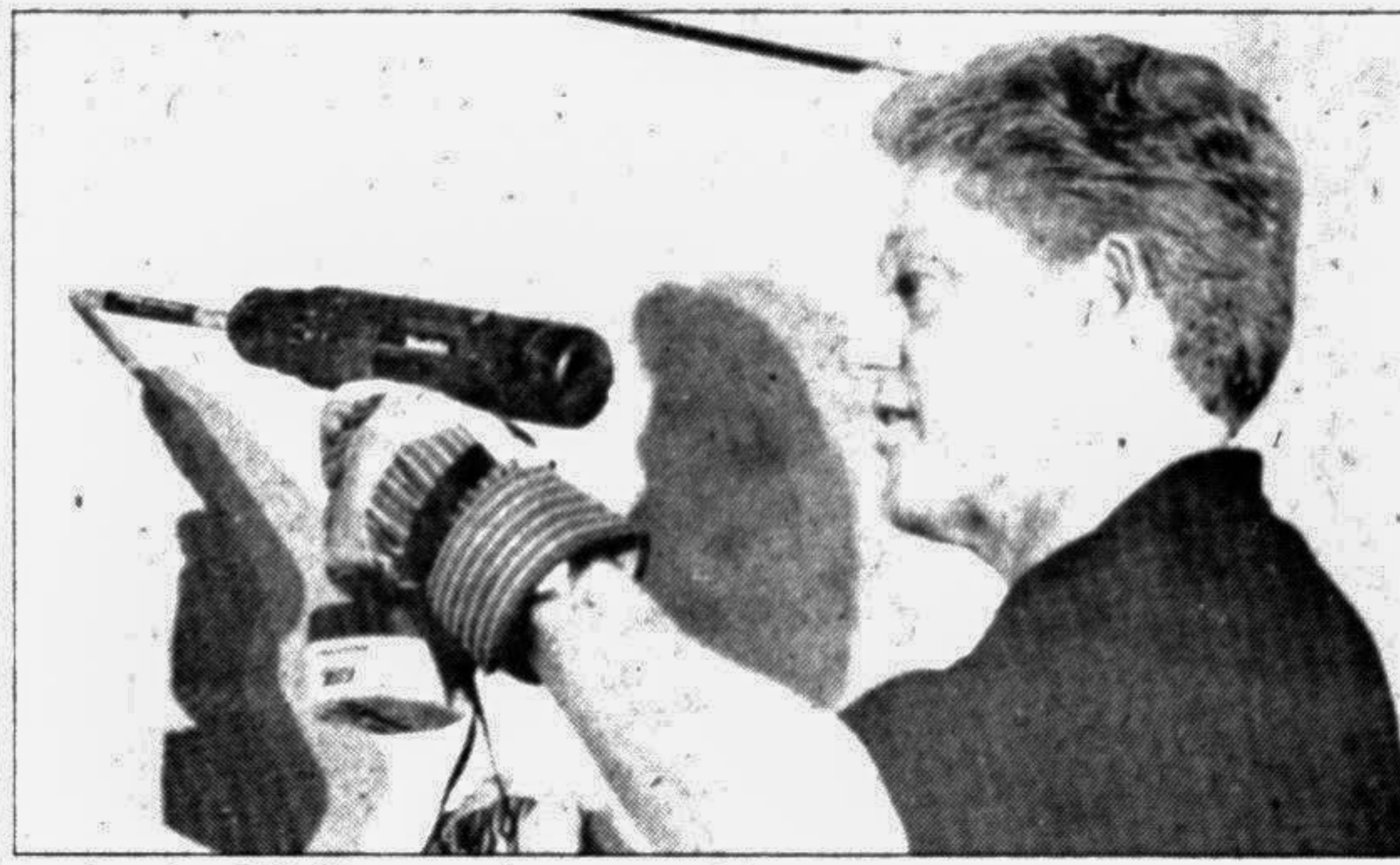
US President Bill Clinton attaches a piece of drywall Monday to the Salem Baptist Church in Fruitland, Tennessee. The church, founded in 1872 and destroyed by suspected arson December 30 1995, is being rebuilt by the community. — AFP/UNB photo
