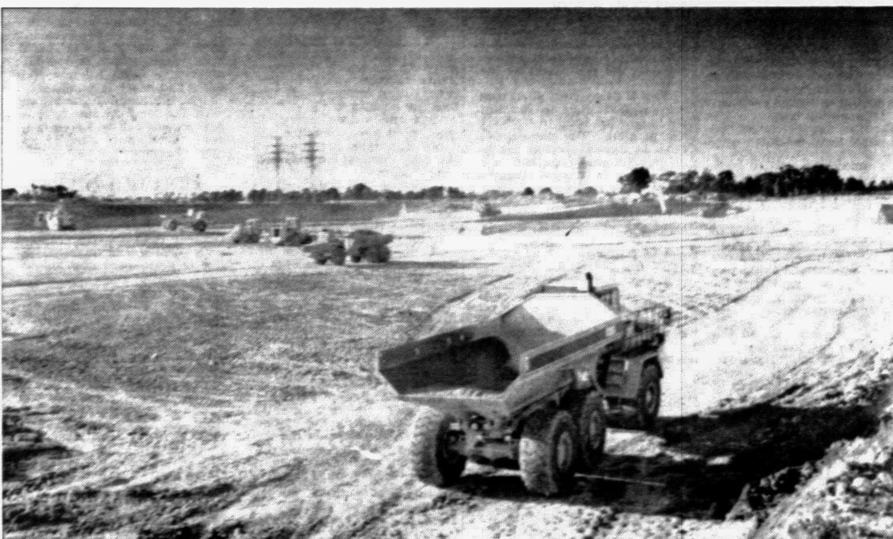
Heavy earthmoving machinery at work on the site of the main Olympic Stadium in Sydney yesterday. The city hosts the 2000 Games. In the background are the controversial, high-voltage electricity pylons the US TV networks want removed before the mega-event gets underway.
