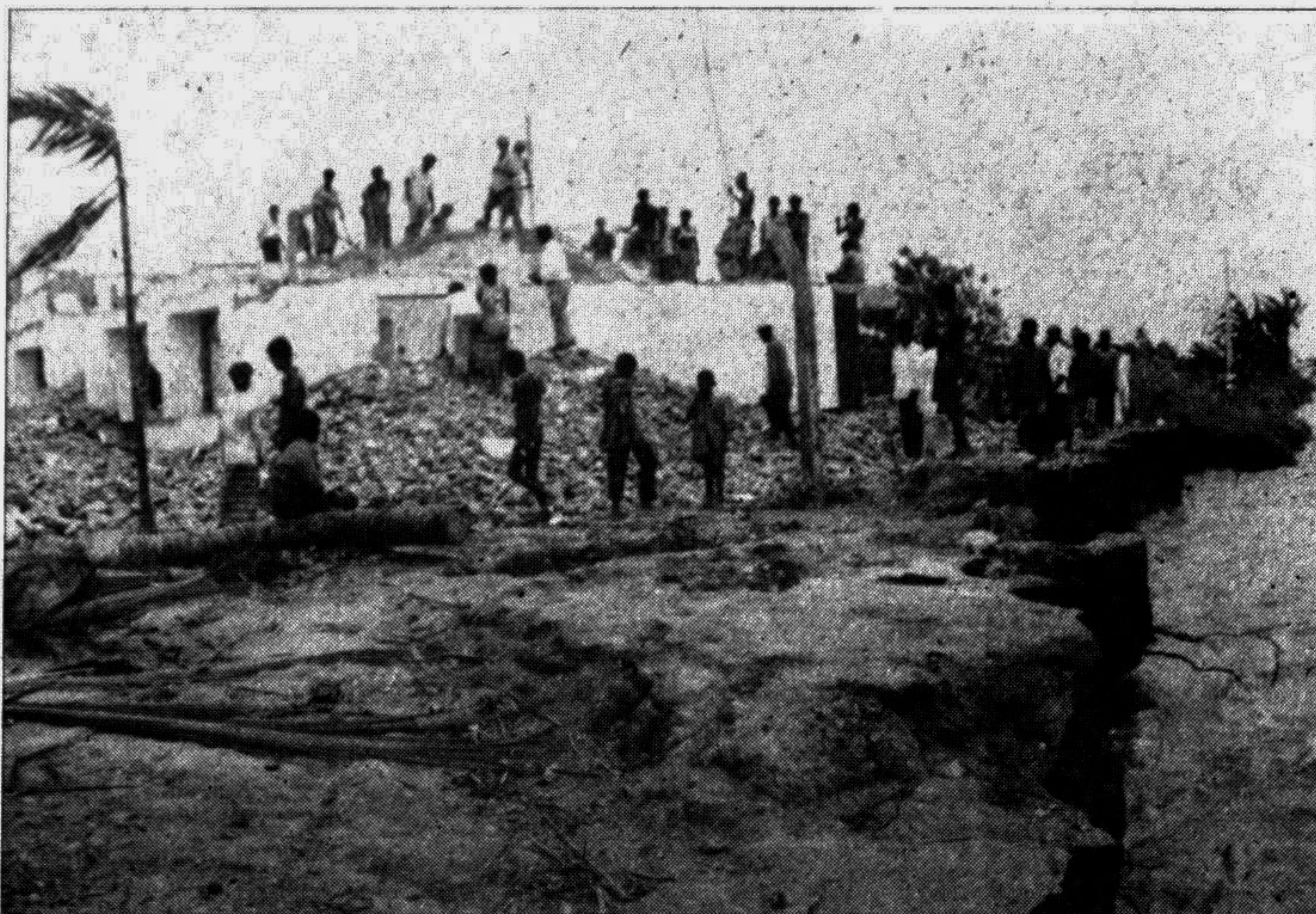
MUNSHIGANJ: Labourers working at the partially eroded building of Dhaida Health Complex in Louhaganj thana of Munshiganj. — Star photo
