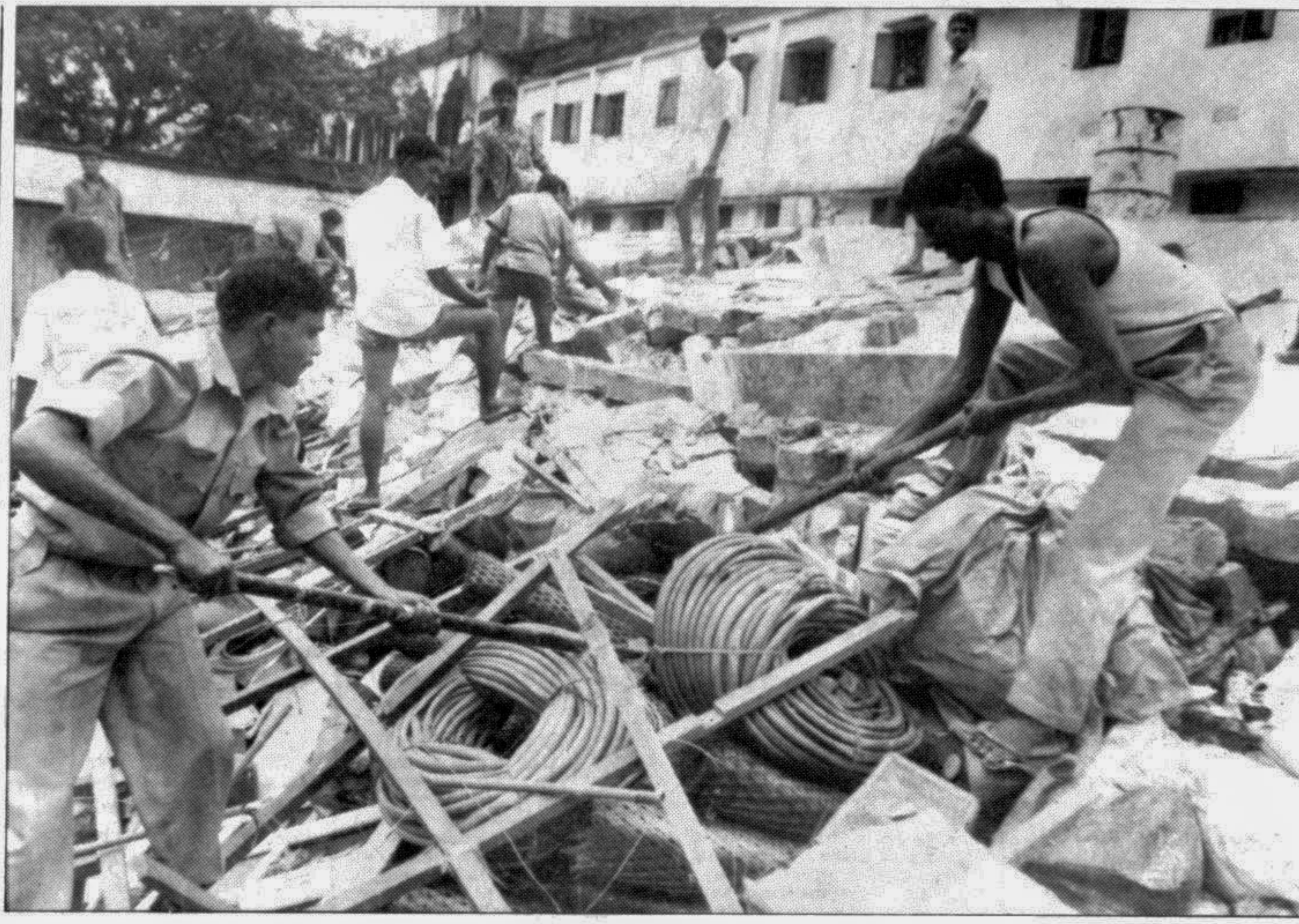
Rescue workers clearing rubbles of a building that collapsed yesterday at Shantinagar in the city.
