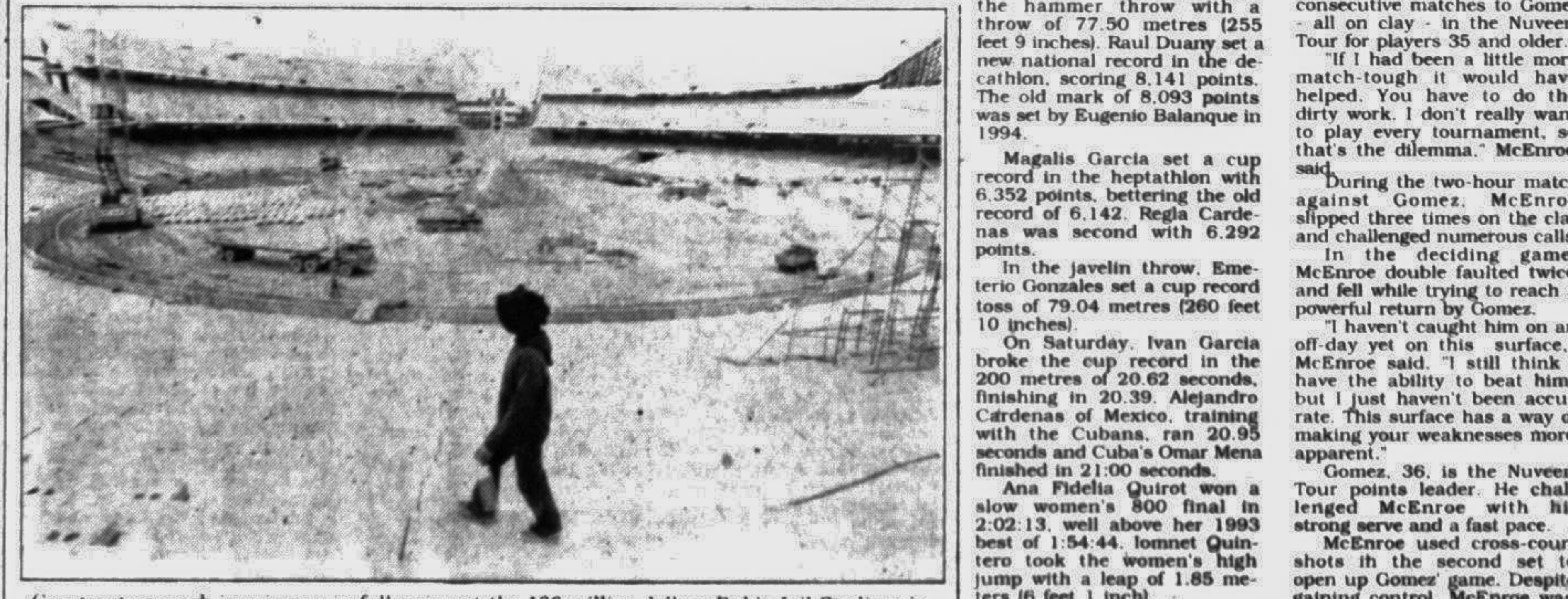
Construction work is going on in full swing at the 136 million dollars Bukit Jalil Stadium in Kuala Lumpur. The stadium is the main venue of the 16th Commonwealth Games due to be held in 1998. — AFP/UNB photo
