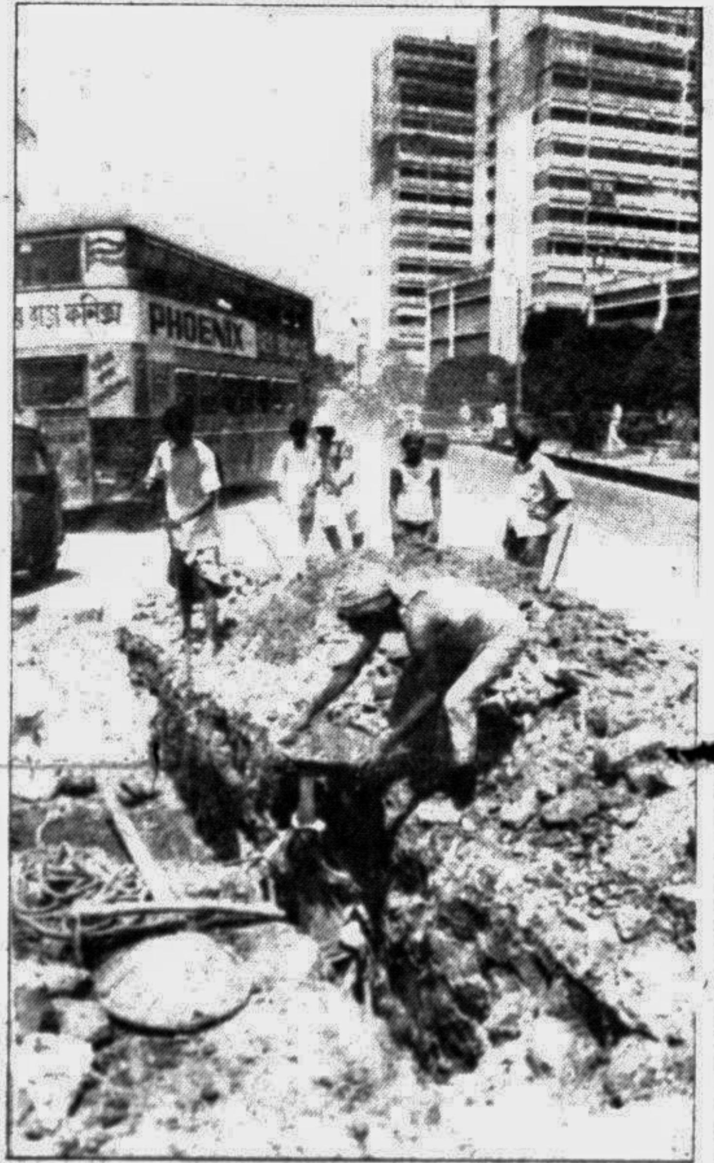
WASA began digging roads in city's busy Shahbag crossing. This picture was taken yesterday. — Star photo
