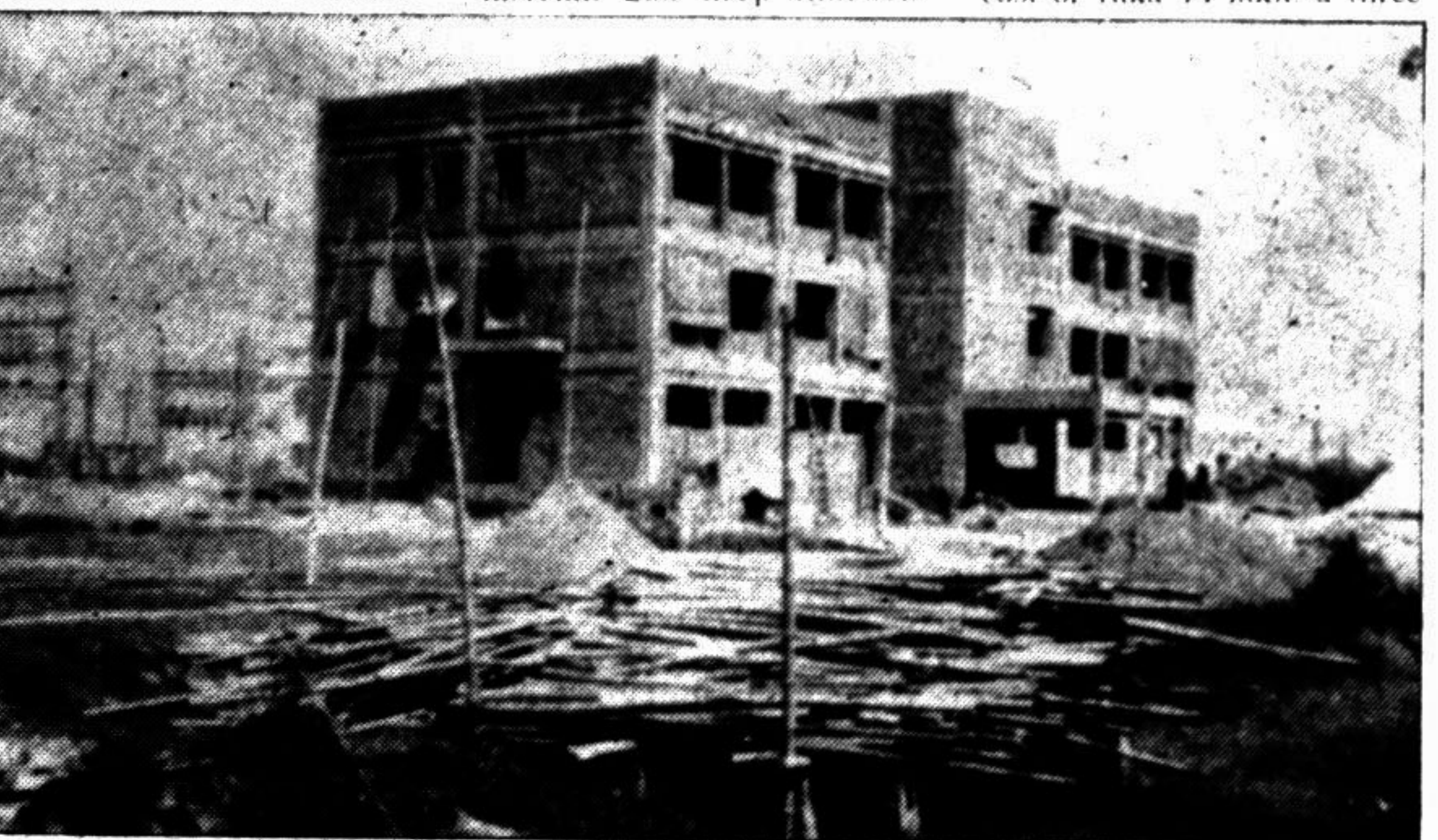
JHENIDAH: Construction work of the REB building at Jhenidah town nearing completion. — Star photo
