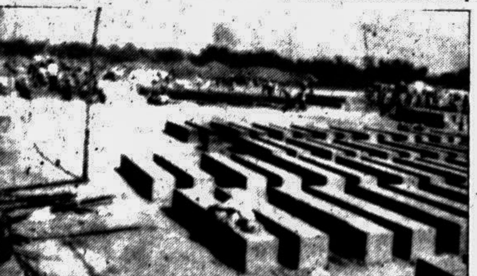
About 2 crore concrete stones have been readied for the embankment. — Star photo
