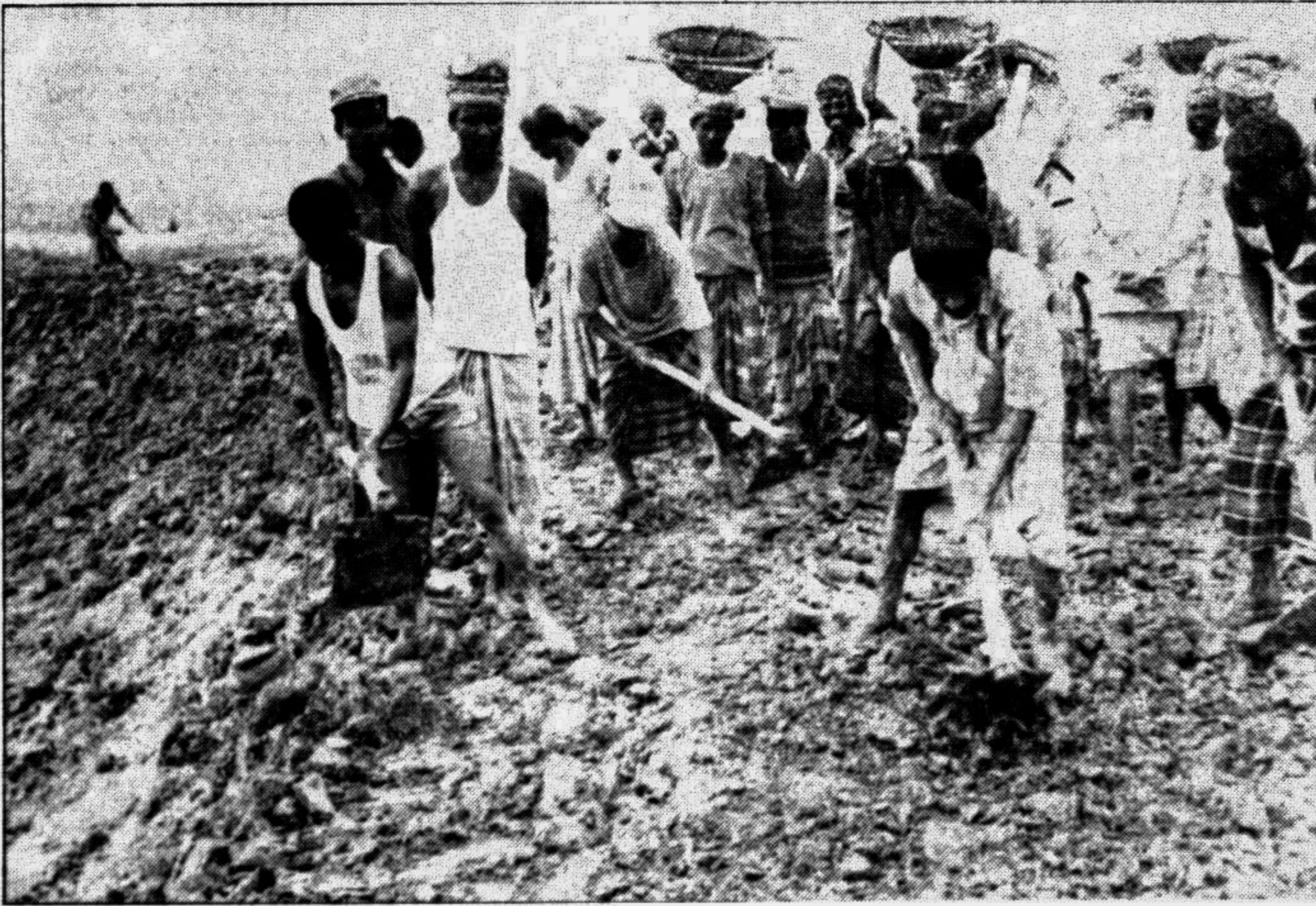
Earth filling work of to be Baligaon-Kalama road is progressing fast in Munshinganj district. This road was totally damaged by the recent flood. — Star photo by Mohsin
