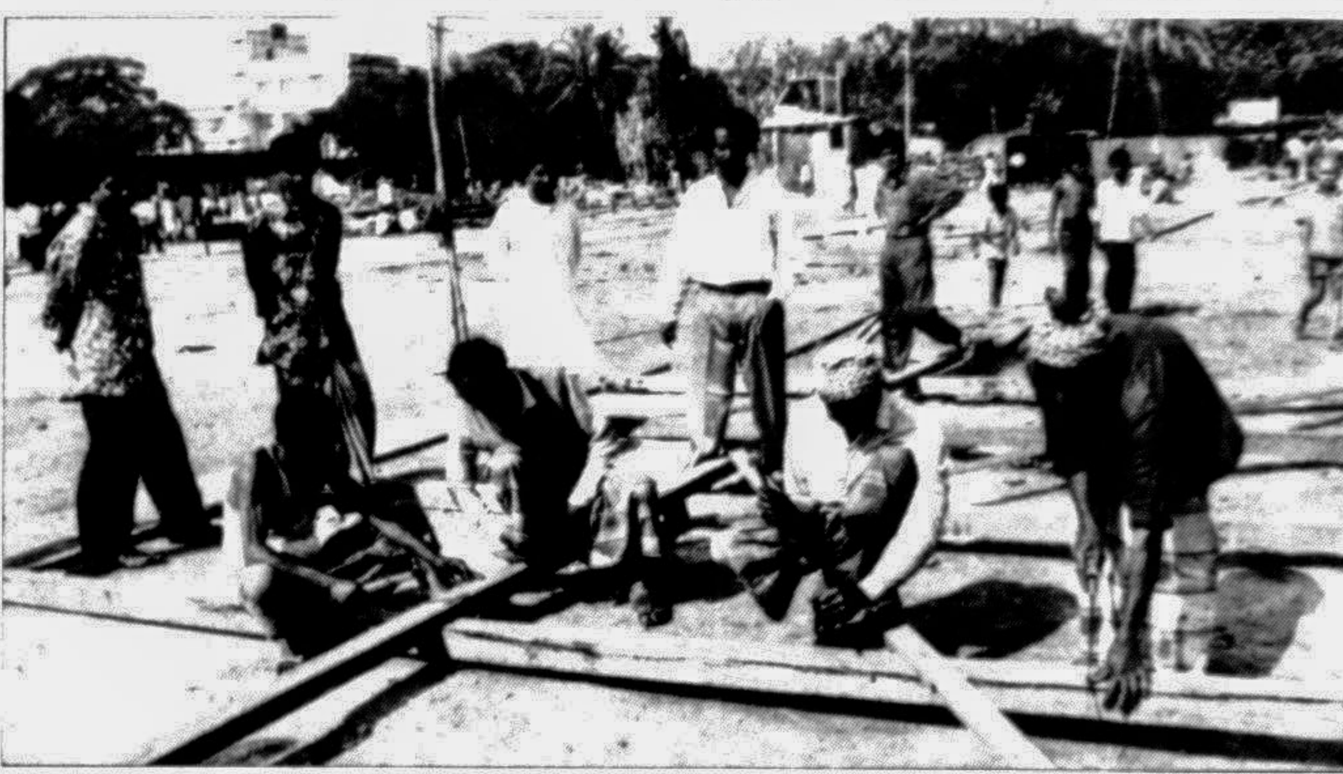
Reconstruction of the gutted Bangabazar in the city has begun. — Star photo
