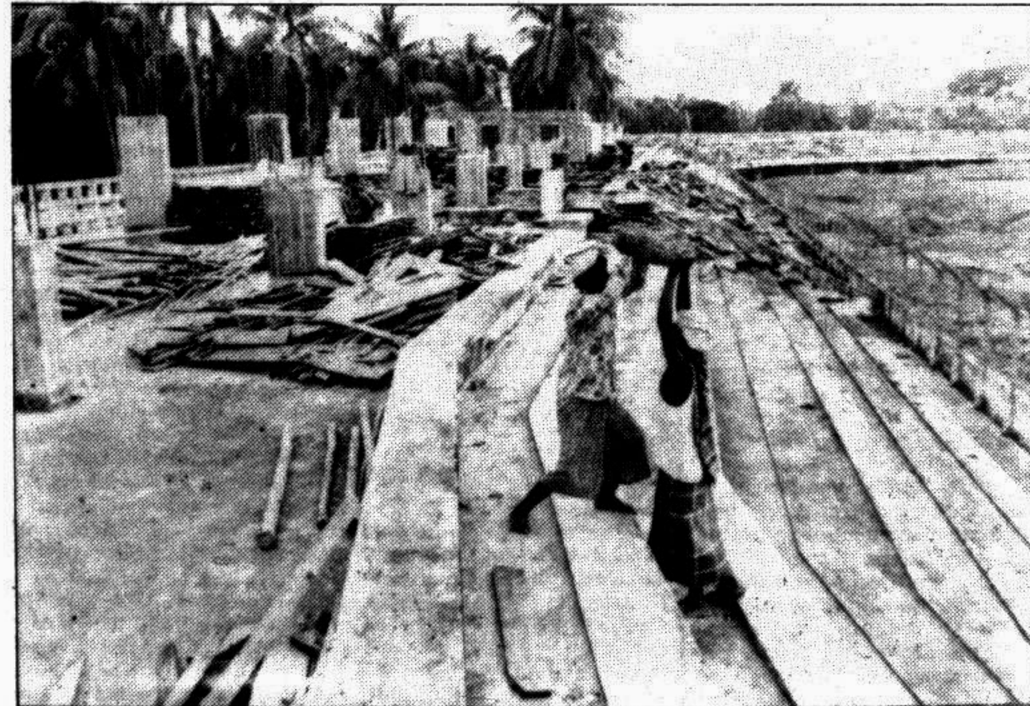
Construction works of the Hockey Stadium gallery in the city is going on at a snail's pace. This photo was taken yesterday. — Star photo by Anisur Rahman
