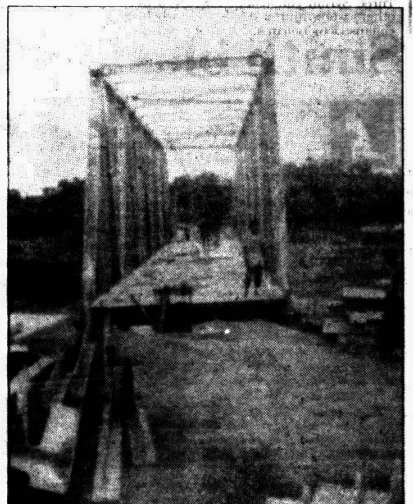
JHENIDAH: Construction work of a baily bridge on river Kumar in Saikupa thana is nearing completion. The project is implemented at a cost of Tk one crore. — Star photo
