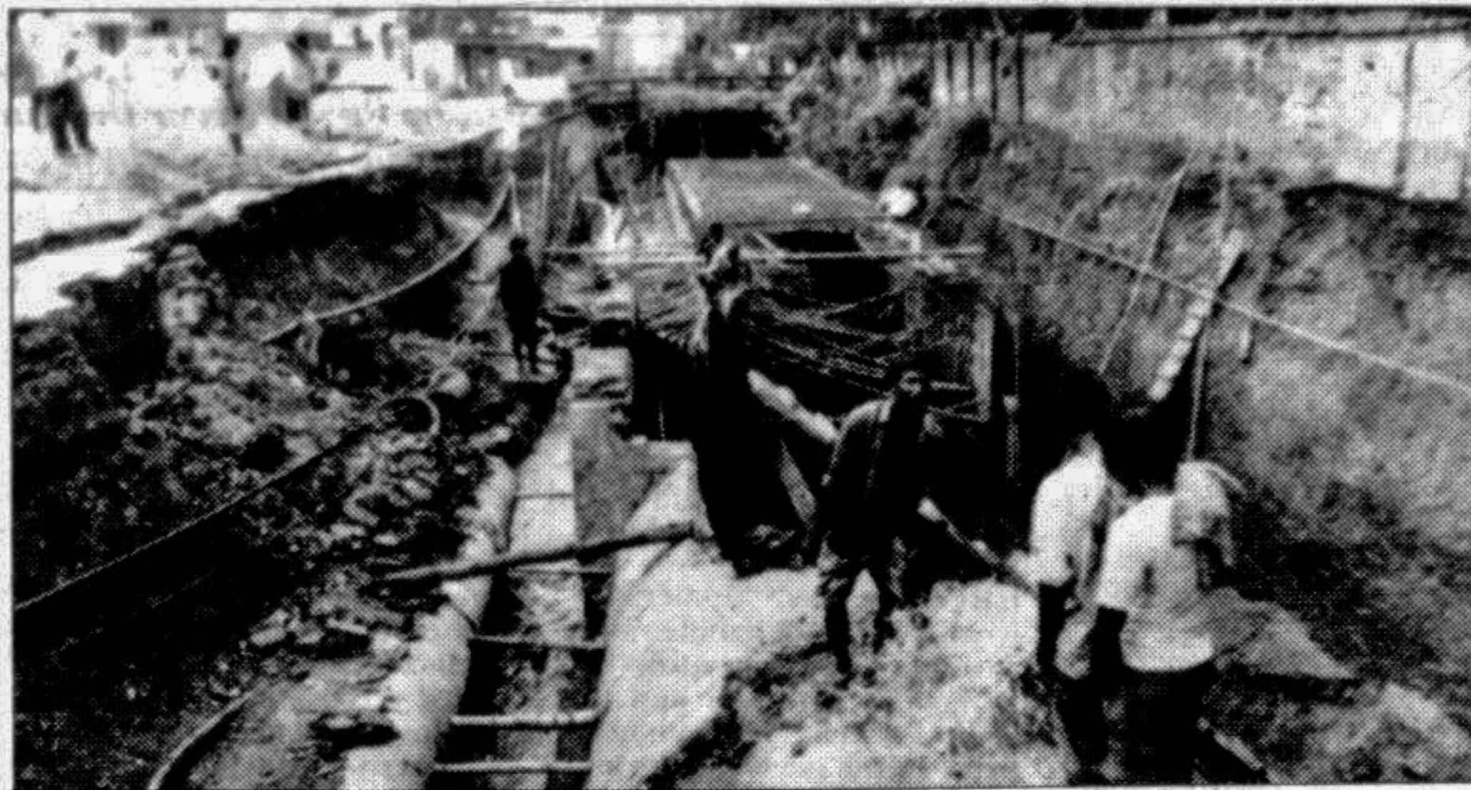
Reconstruction of sewerage line in city's Hatirpool area is in progress. This picture was taken yesterday. — Star photo
