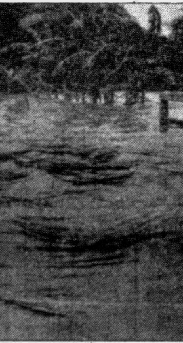
JAMALPUR: Flood inundated Melandah-Madarganj-Sharishabari road. Flood water on the road ranges from two to seven feet deep. Fifty-five bridges and culverts have been washed away in the recent flood.
