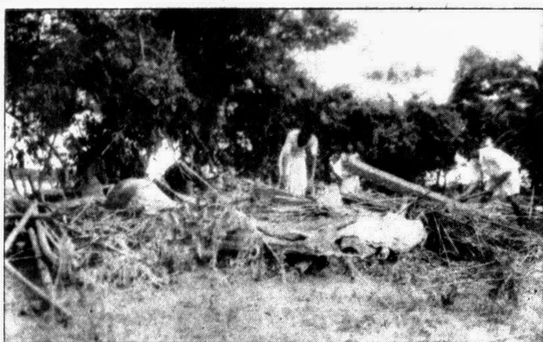
SYLHET: With the recession of flood water, most of the villagers have started to come back. Some villagers of Uttar Kholachhara under Companyganj thana rebuilding their thatched house. — Star photo
