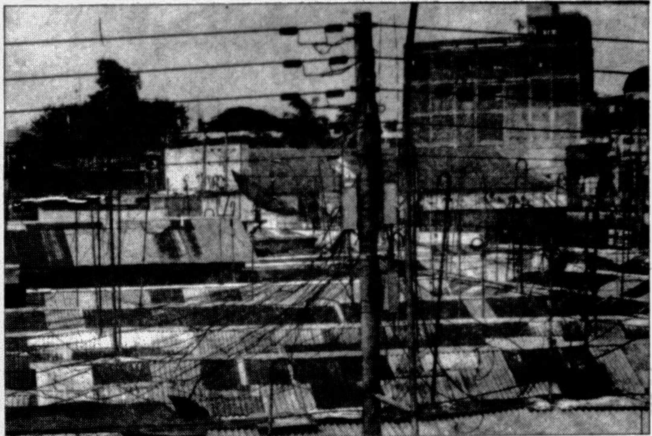
Such connections, from a single electricity pole, always pose a serious risk to life and property in the city. This picture was taken at Shyamoli yesterday. — Star photo
