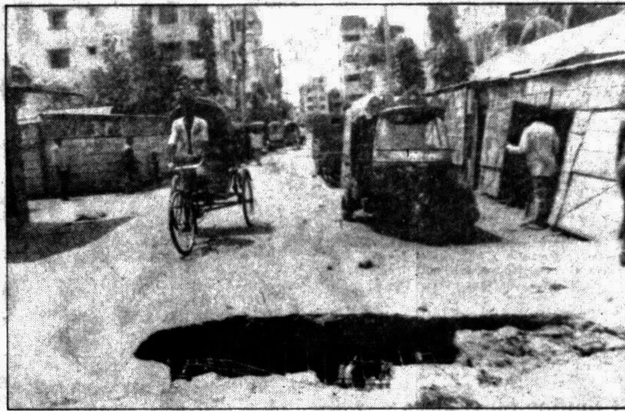
This big pothole in the city's Khilgaon Sipahibagh Road has been left unrepaired for quite sometime now. — Star photo
