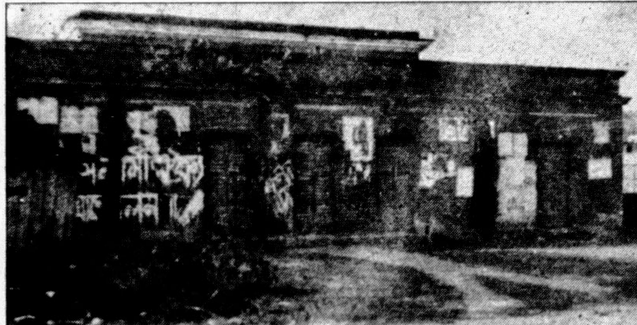
GAIBANDHA: An age old building situated at old collectorate area might collapse at any time. The building is being used by some employees of the union offices. — Star photo
