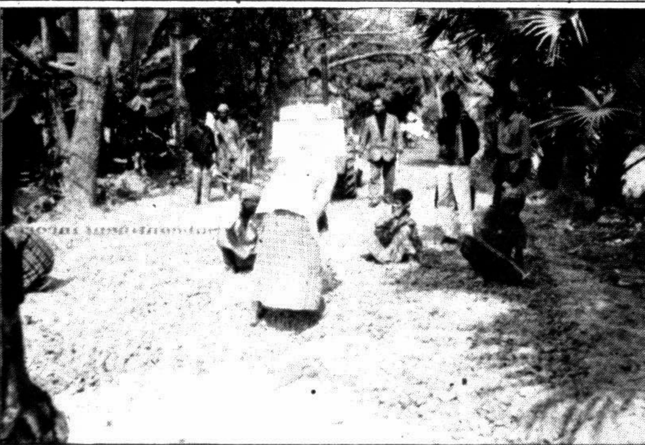
JHENIDAH: An ASS and DBST road being constructed between Hatgopalpur and Narkelbaria under Jhenidah sadar thana of the district. — Star photo
