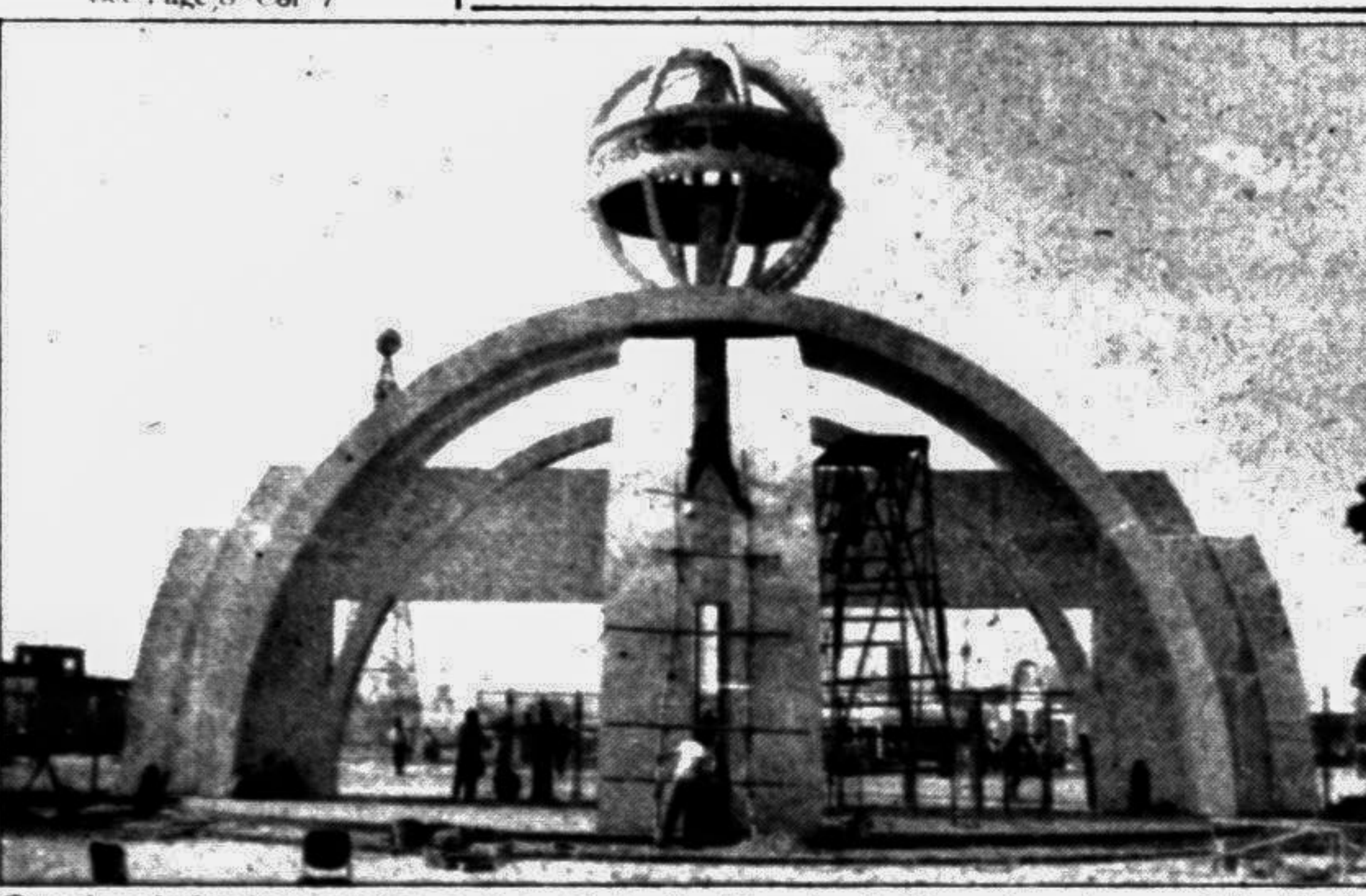
Two days before its opening, workers giving final touches to the main entrance of the Dhaka International Trade Fair '95 at Sher-e-Bangla Nagar yesterday. — Star photo
