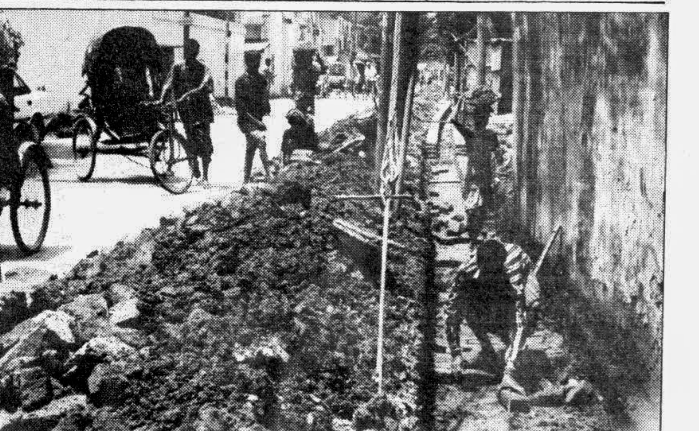
The renovation and repairing work of drains at city's Segunbagicha area is on progress amidst the rains. —Star photo
