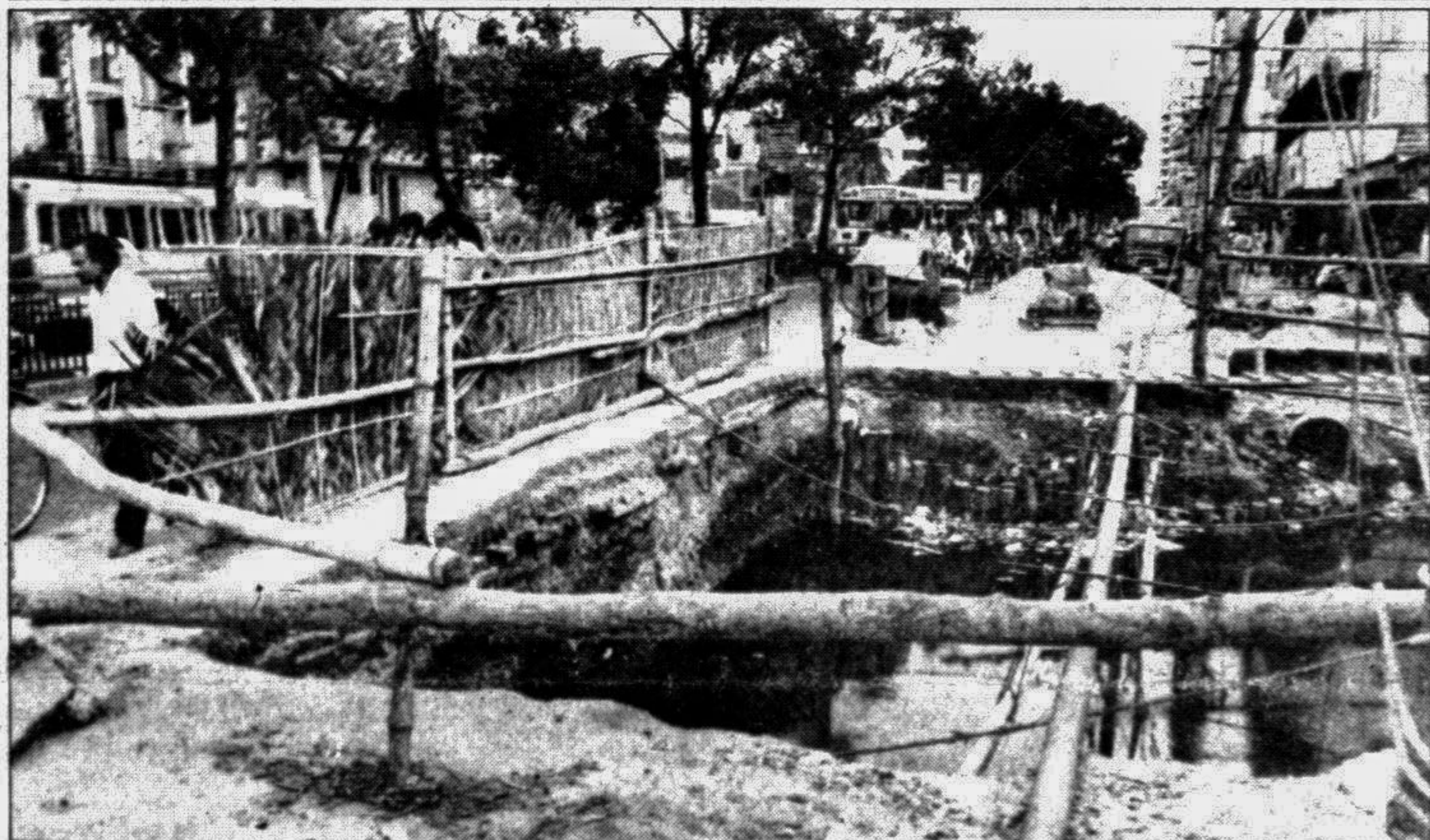
This gaping hole on the Bijoynagar Road, dug sometime ago for development works by a government agency, now awaits the onslaught of the monsoon rains. — Star photo
