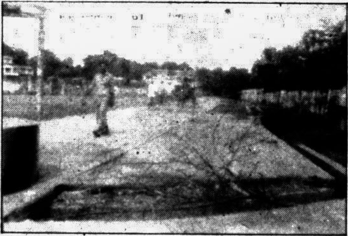
GOPALGANJ: A damaged part of Stadium Road of the town has been covered by branches of trees for a long time. — Star photo
