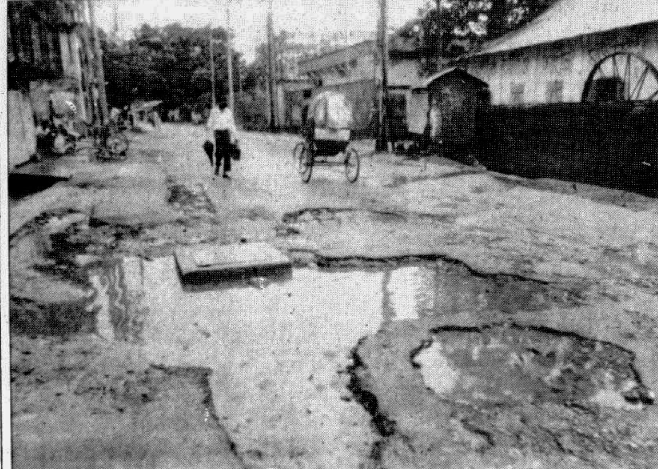
SYLHET: The dilapidated condition of a road in the town. — Star photo
