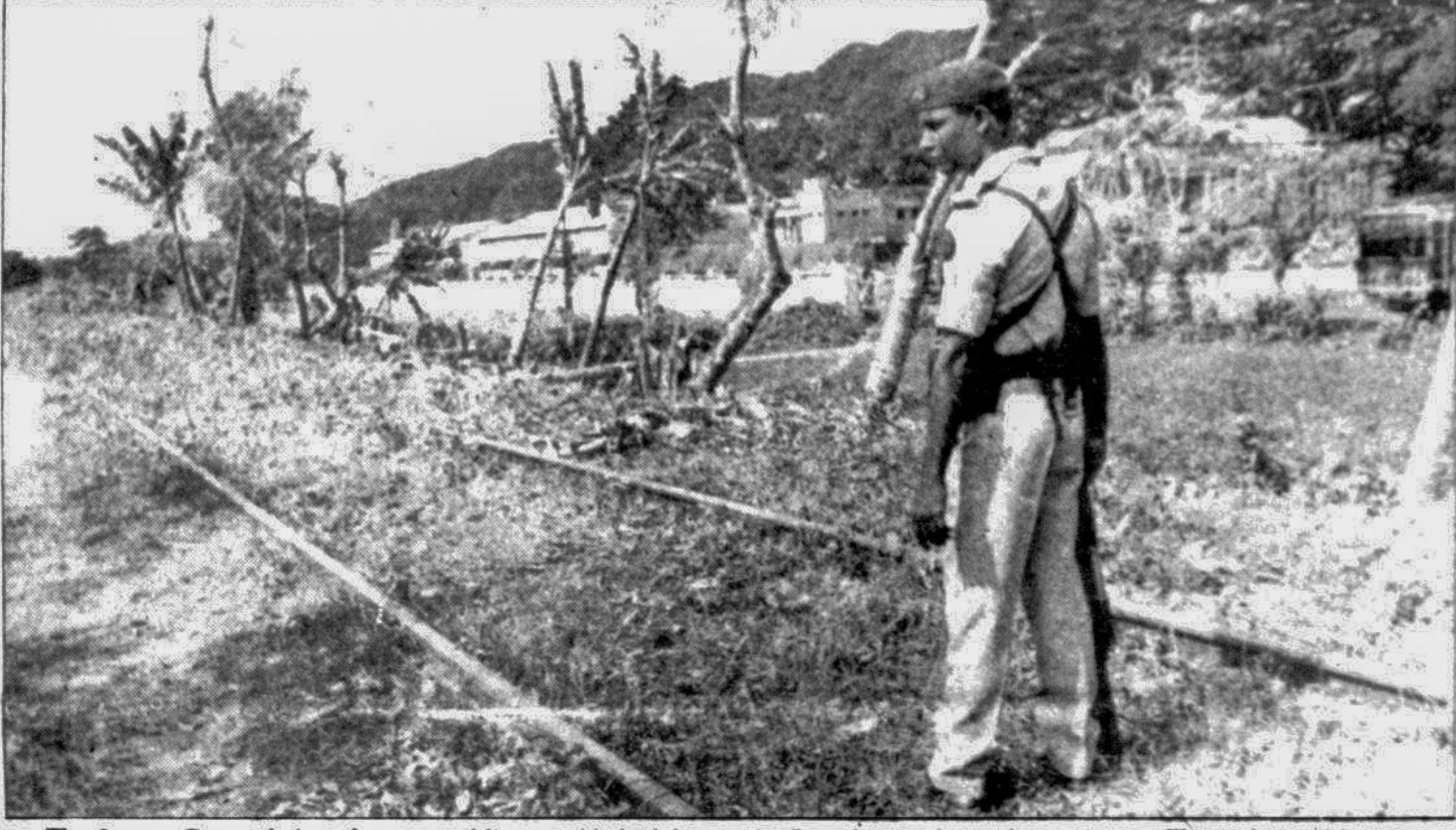
The Jessore-Benapole broad gauge rail line established during the British period is no longer in use. The 34-km rail line can be made fully operational with a repair work costing around Tk 5 crore, experts say. Observers believe that this will help facilitate transportation of goods between Jessore and Benapole as well as carrying of coal and limestones from India. — Star photo by AKM Mohsin
