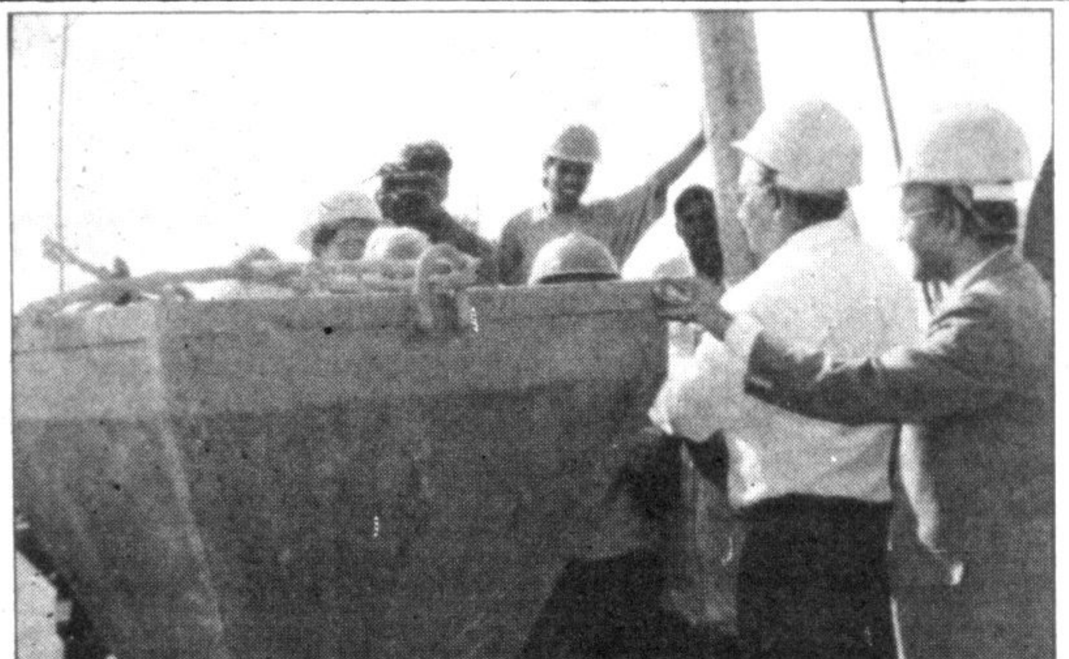
Finance Minister M Saifur Rahman inaugurating the piling work of Sylhet 90 MW Combined Cycle Power Plant Project at Fenchuganj on Nov 25. Energy and Mineral Resources Minister Dr Khondaker Mosharraf Hossain is seen in the picture.
