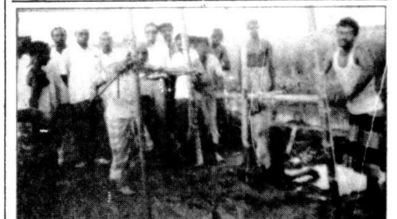
SYLHET: Test boring of a deep tubewells began at Tetli village of Sylhet sadar thana under the national small irrigation project recently. The picture shows installation of the deep tubewell. — Star photo
