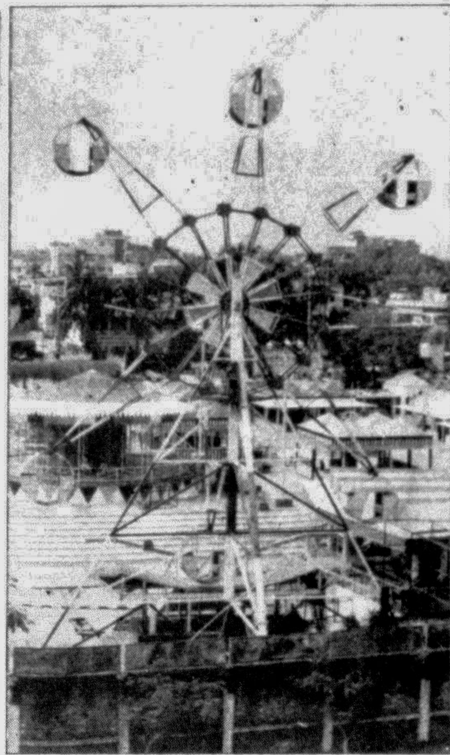
View of an under-construction private sector children's and amusement park near the Orthopaedics (Pangu) Hospital at Shyamoli in the city. — Star photo
