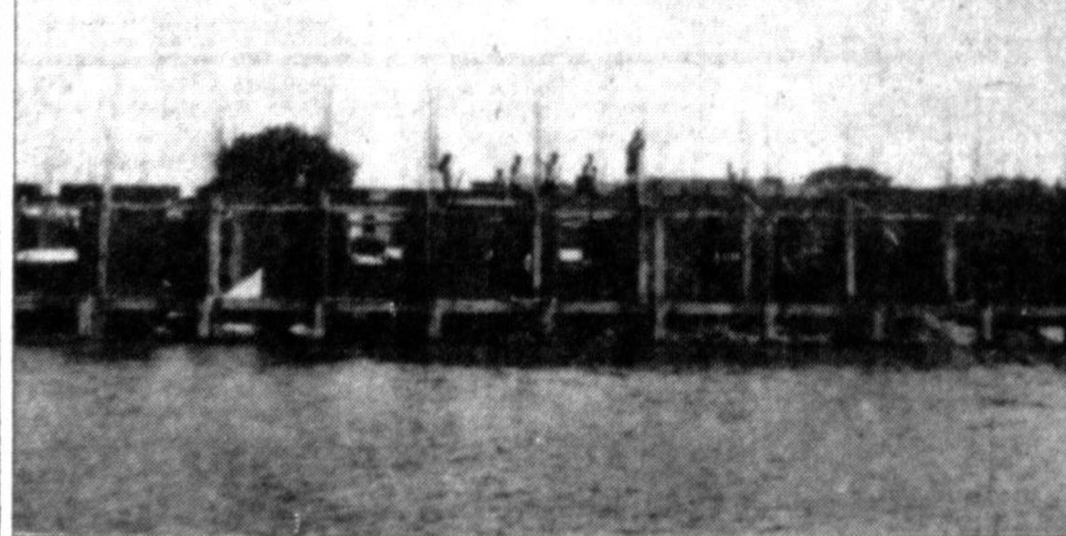
CHANDPUR: The building of Raymunessa Women's College at Matlab thana is under construction. — Star photo
