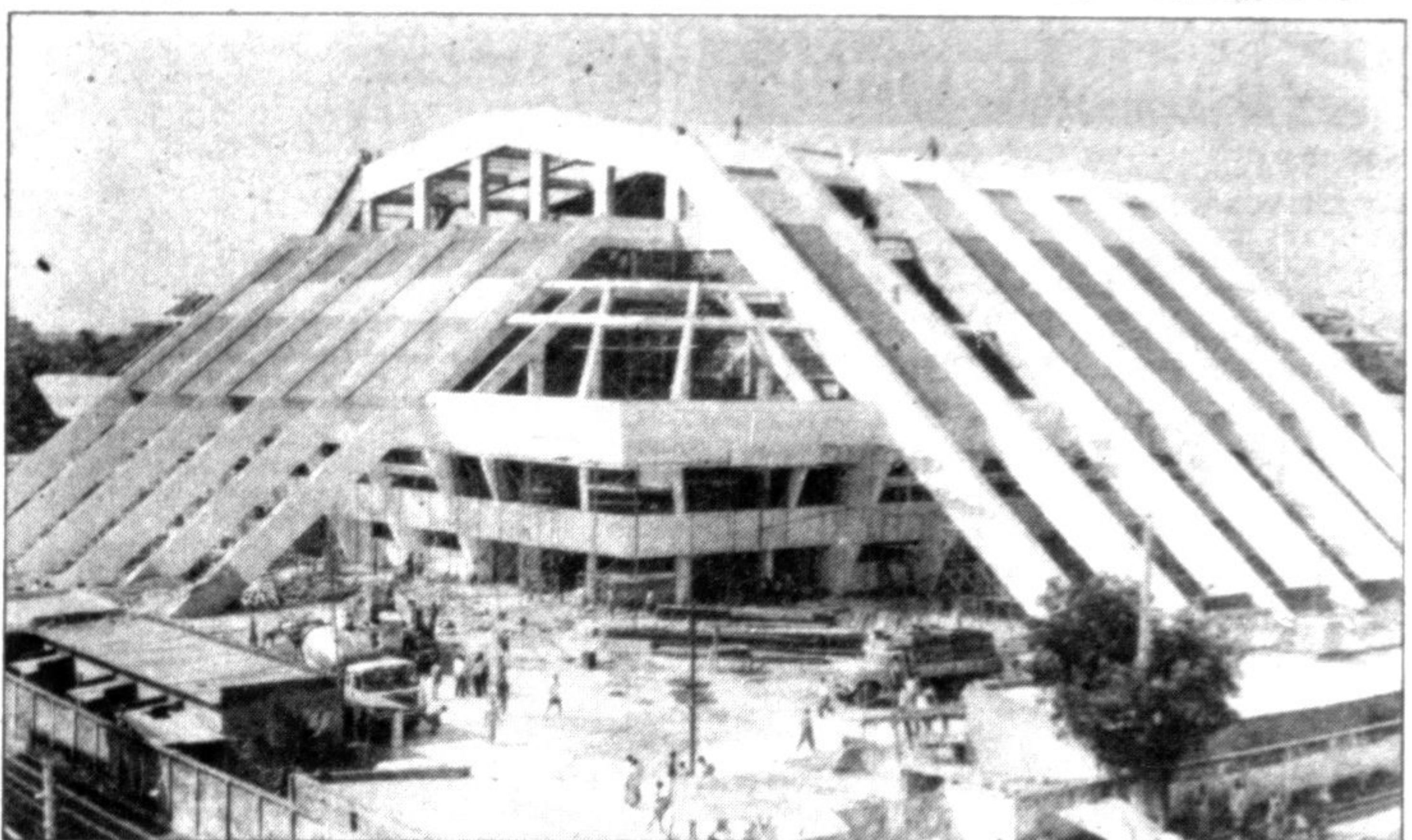
Construction of a modern indoor stadium at Mirpur, to be used during next month's 6th SAF Games December 20-27, is going on in full swing. —Star photo
