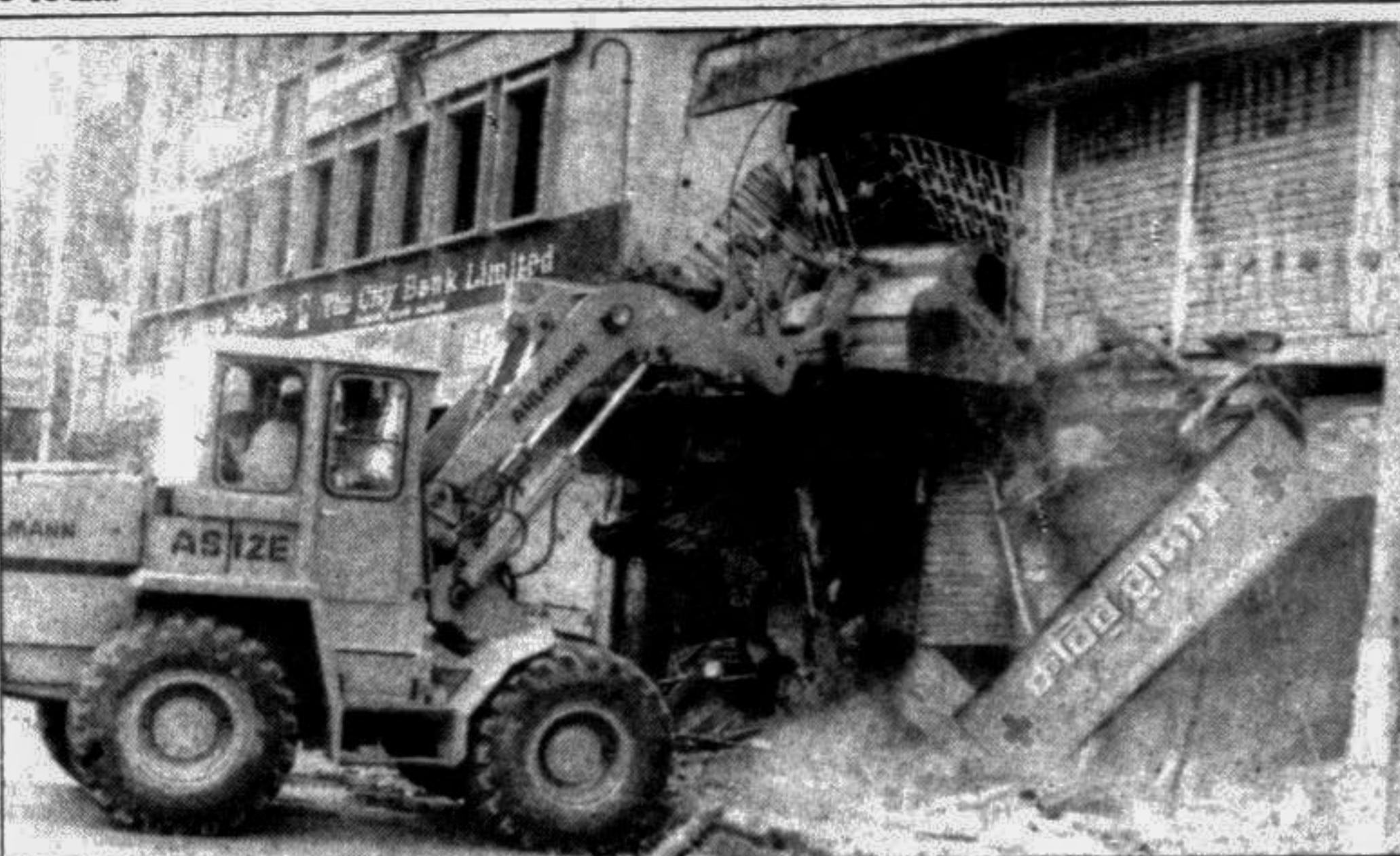
Some unauthorised constructions near Malibagh crossing in the city were demolished by the authorities yesterday. —Star photo
