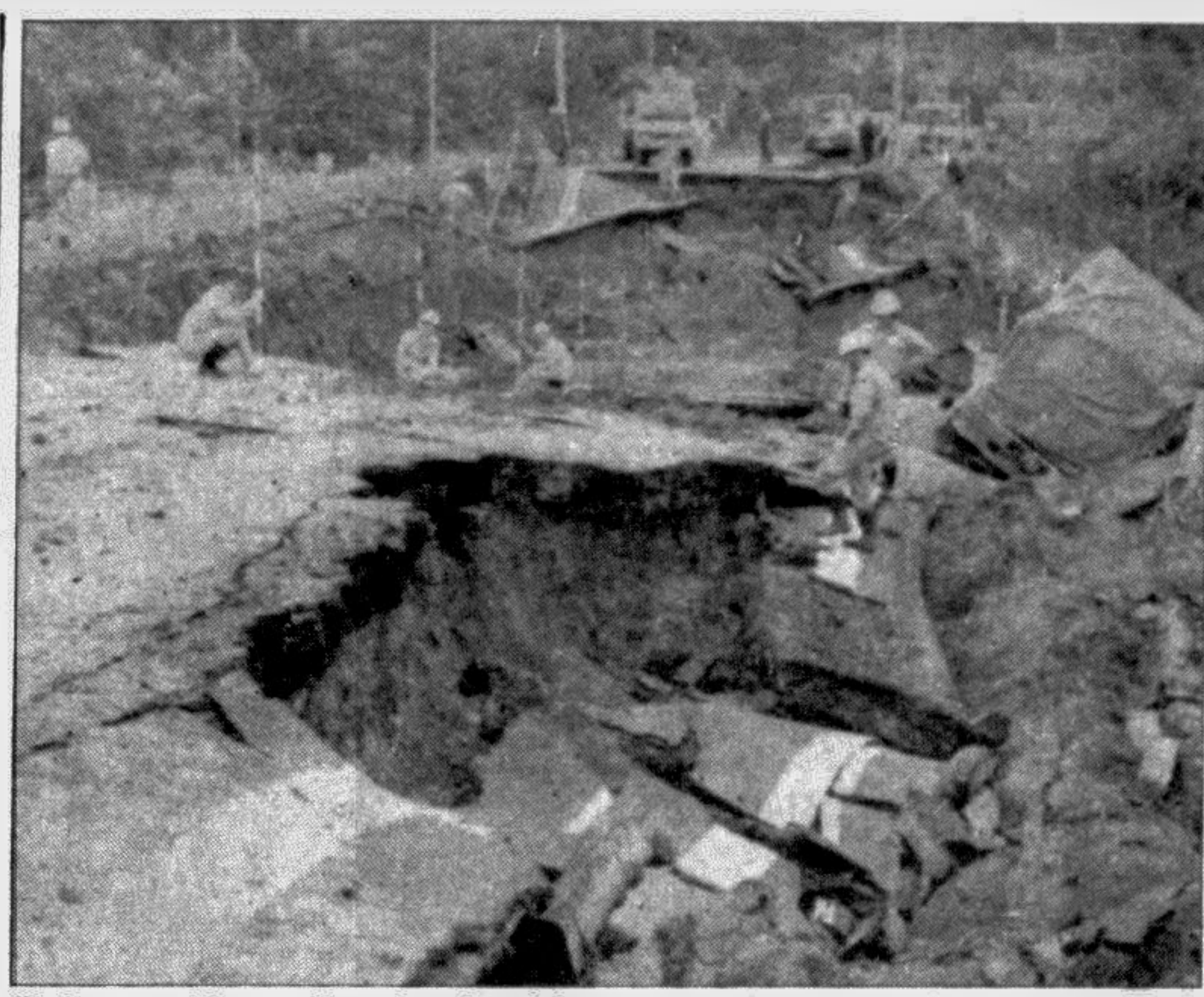
Workers repairing a collapsed road in Oshamanoe, 100 km north of Hakodate (Hokkaido island) in Japan yesterday. A strong earthquake hit extensive areas of Hokkaido and northern Honshu during Monday night.
