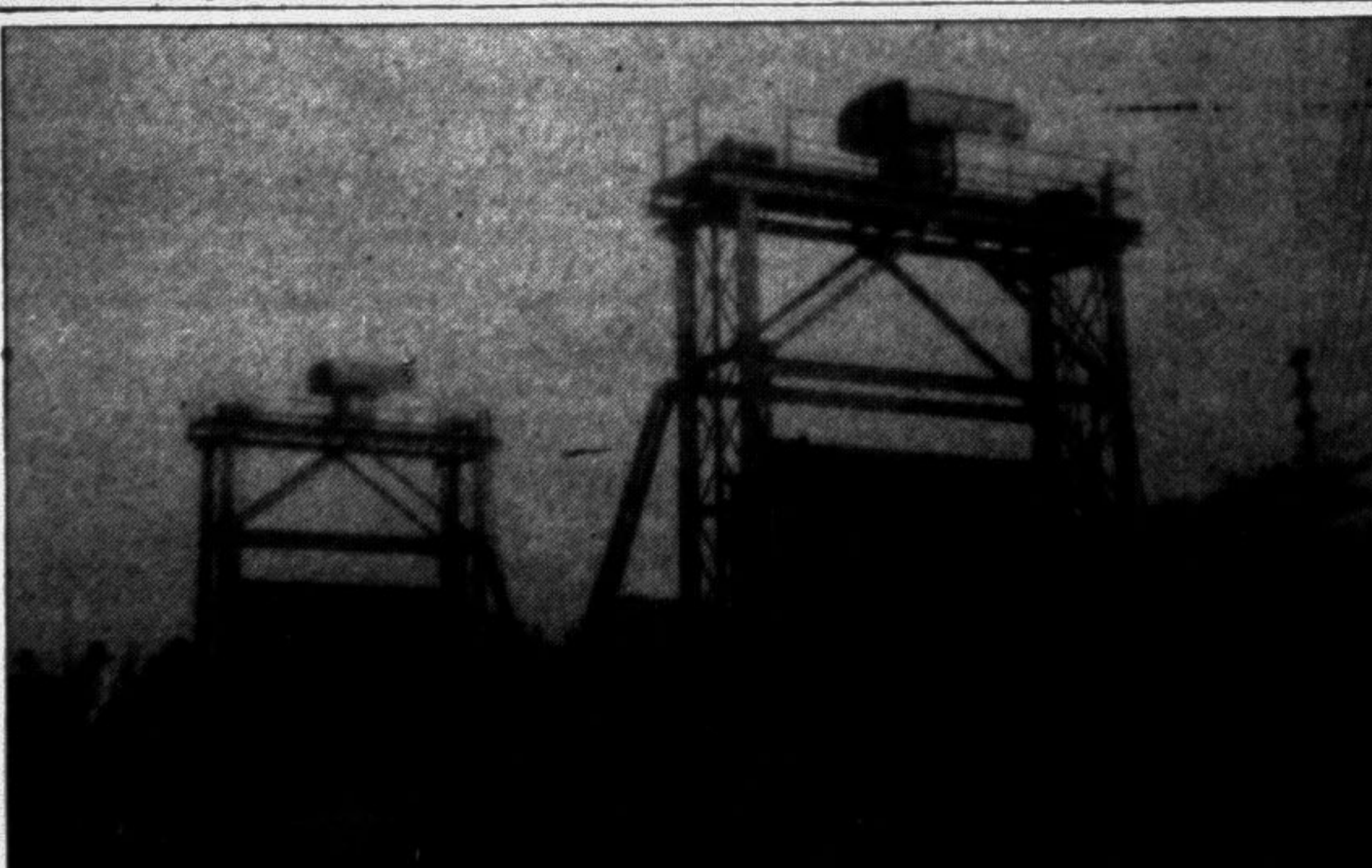
This gigantic looking figure is the 'Lock Gate' as the locals call it. This gate was built during the British rule in this sub-continent to save Gopalganj district from over flow of water from river Madhumati. The whole structure is made of iron. Lack of maintenance has lead to severe rusting. —Star photo
