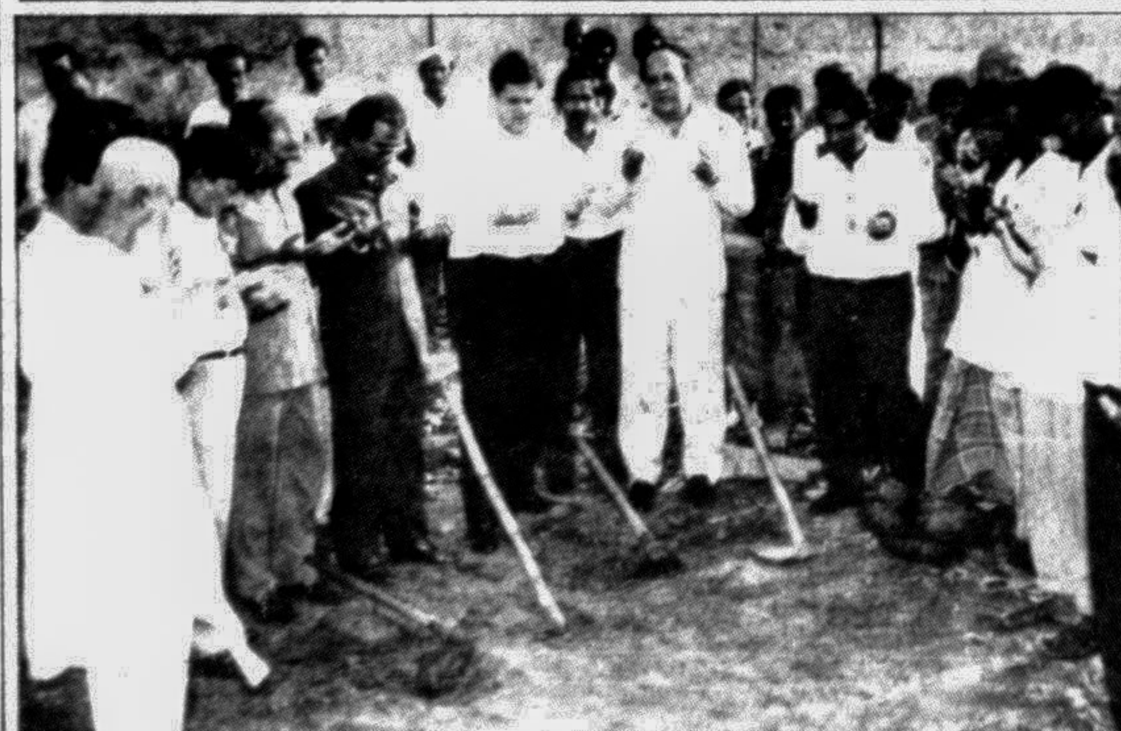
Construction work of the Dhaka Sheraton Hotel's six storey office cum shopping complex got underway recently. John L Eaton, General Manager of the hotel, Shafiqul Bari, Secretary, BSL and cabinet members of the hotel's employee union took part in a milad mahfil on this occasion.
