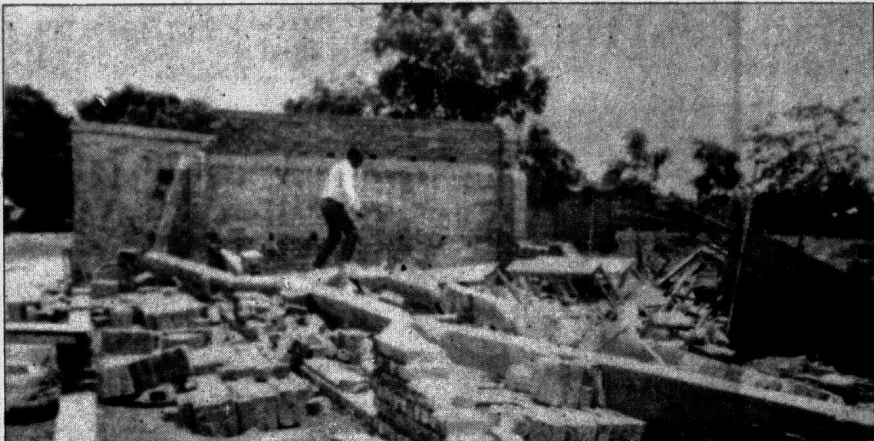
JESSORE: The Patibila Haji Shahjahan Ali High School of Chowgacha thana was badly damaged by the severe cyclonic storm that lashed the district recently. It has not yet been reconstructed causing much inconvenience to the students. —Star Photo
