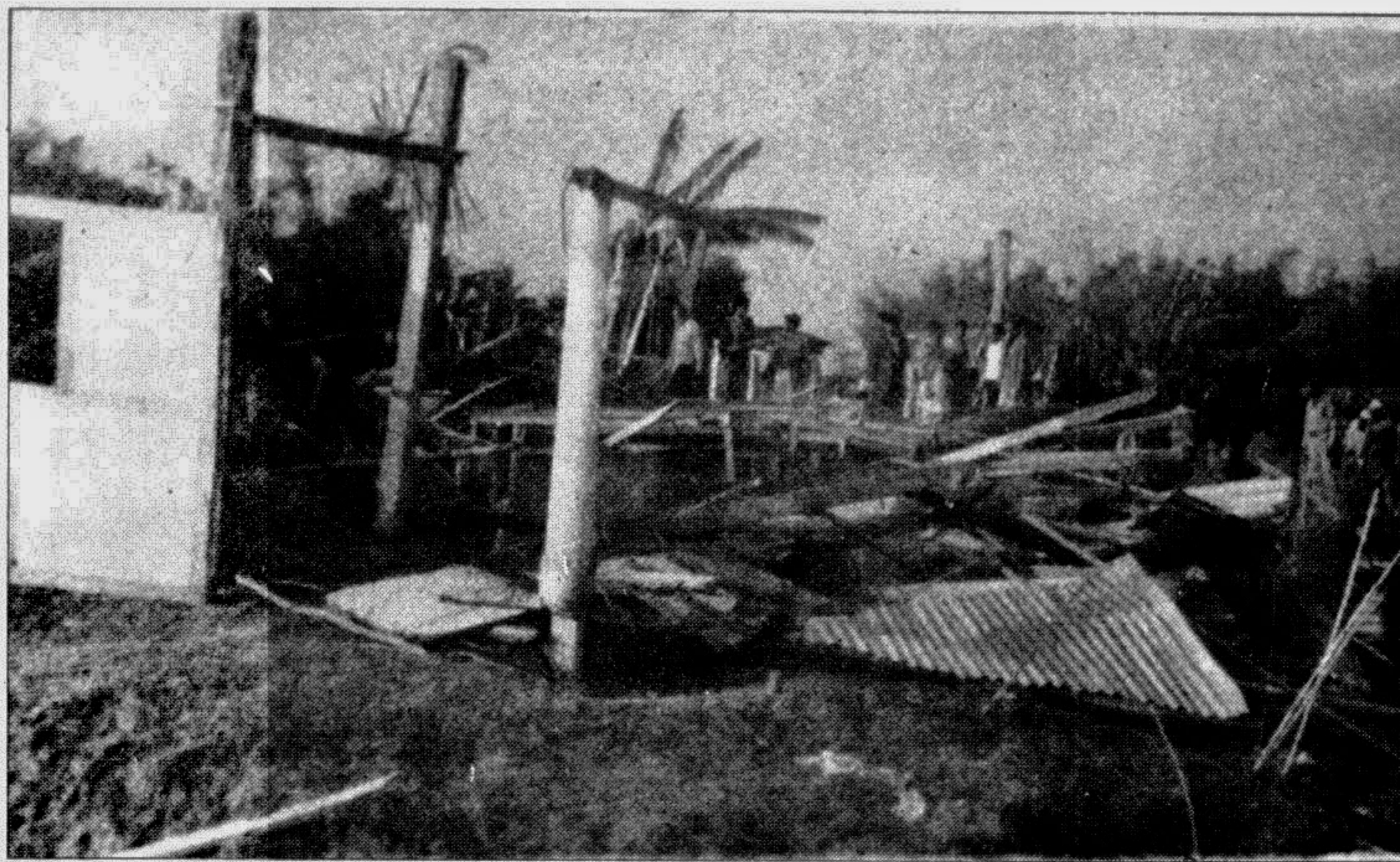
SYLHET: The high school of Gowainghat thana was badly damaged by the severe cyclonic storm that lashed the district in January last has not yet been reconstructed causing much inconveniences to the students. — Star photo
