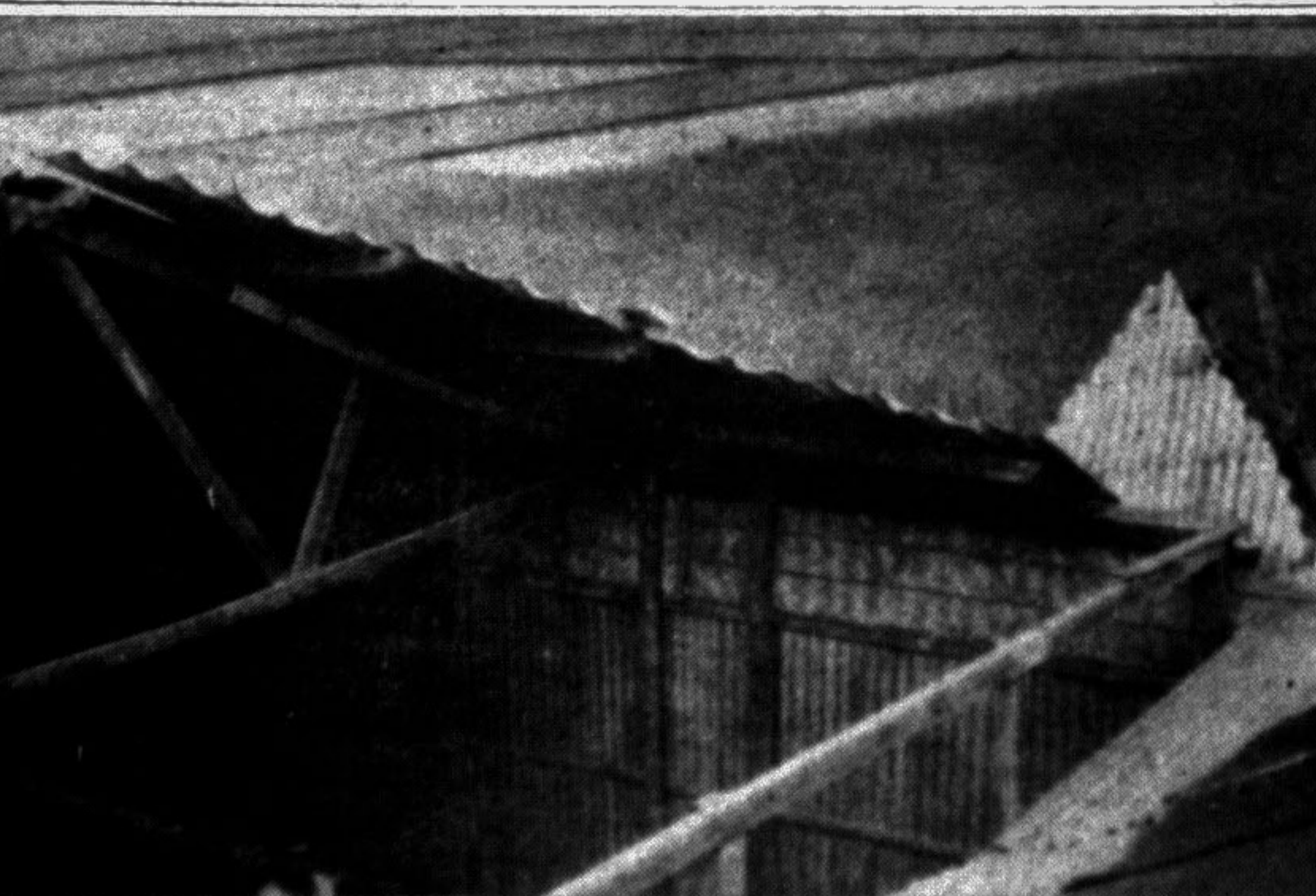
JAMALPUR: Shadupur High School of the district needs early reconstruction. The school was damaged by a recent cyclone. — Star photo
