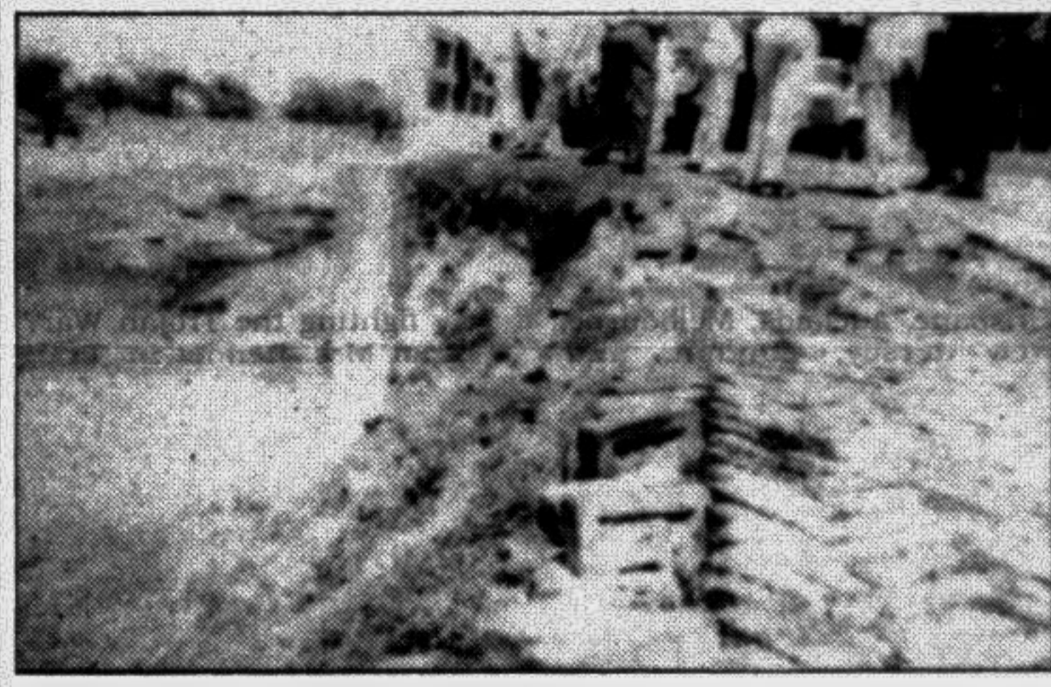
MADARIPUR: The Shibchar-Madaripur road is in pitiable condition which needs immediate repair. —Star photo
