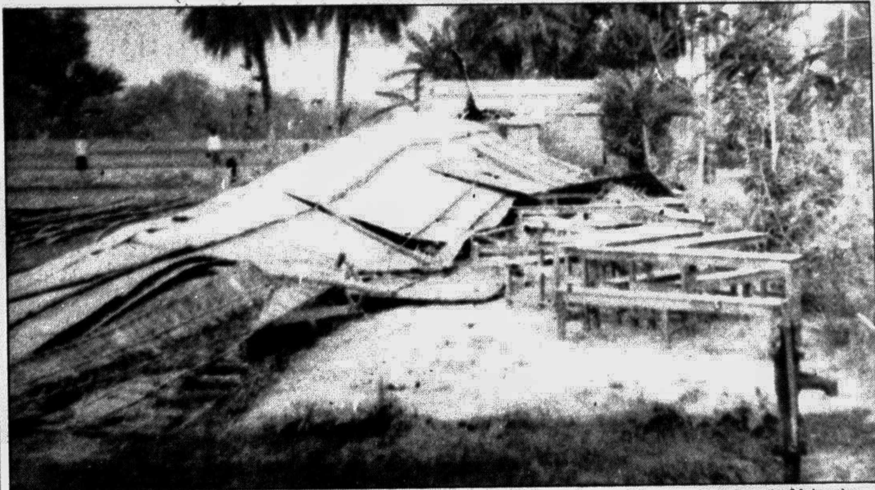
JAMALPUR: Kuna Maluncha Amena Dhakil Madrasha has completely been damaged by recent cyclone in Maluncha thana of the district. — Star photo
