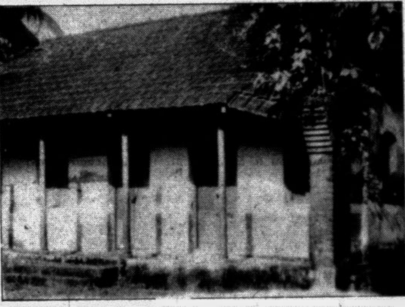
SYLHET: Pitiable condition of one of the government offices in Sylhet town which need immediate reconstruction. — Star photo
