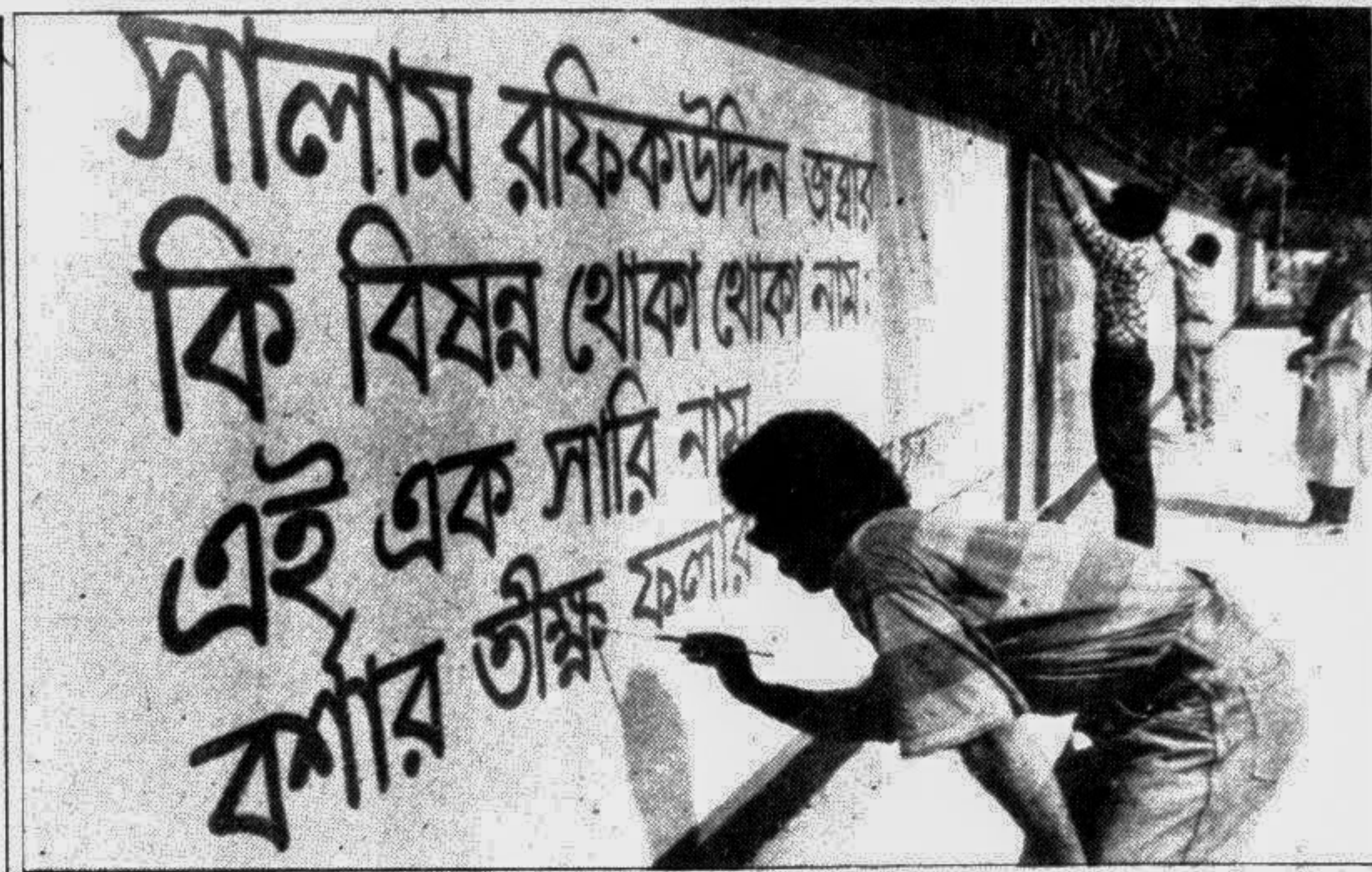
Painters giving a finishing touch to the wall facing the Central Shaheed Minar by inscribing names of martyrs of the Language Movement and quotes from patriotic poems in preparation of the Amar Ekushey. — Star photo
