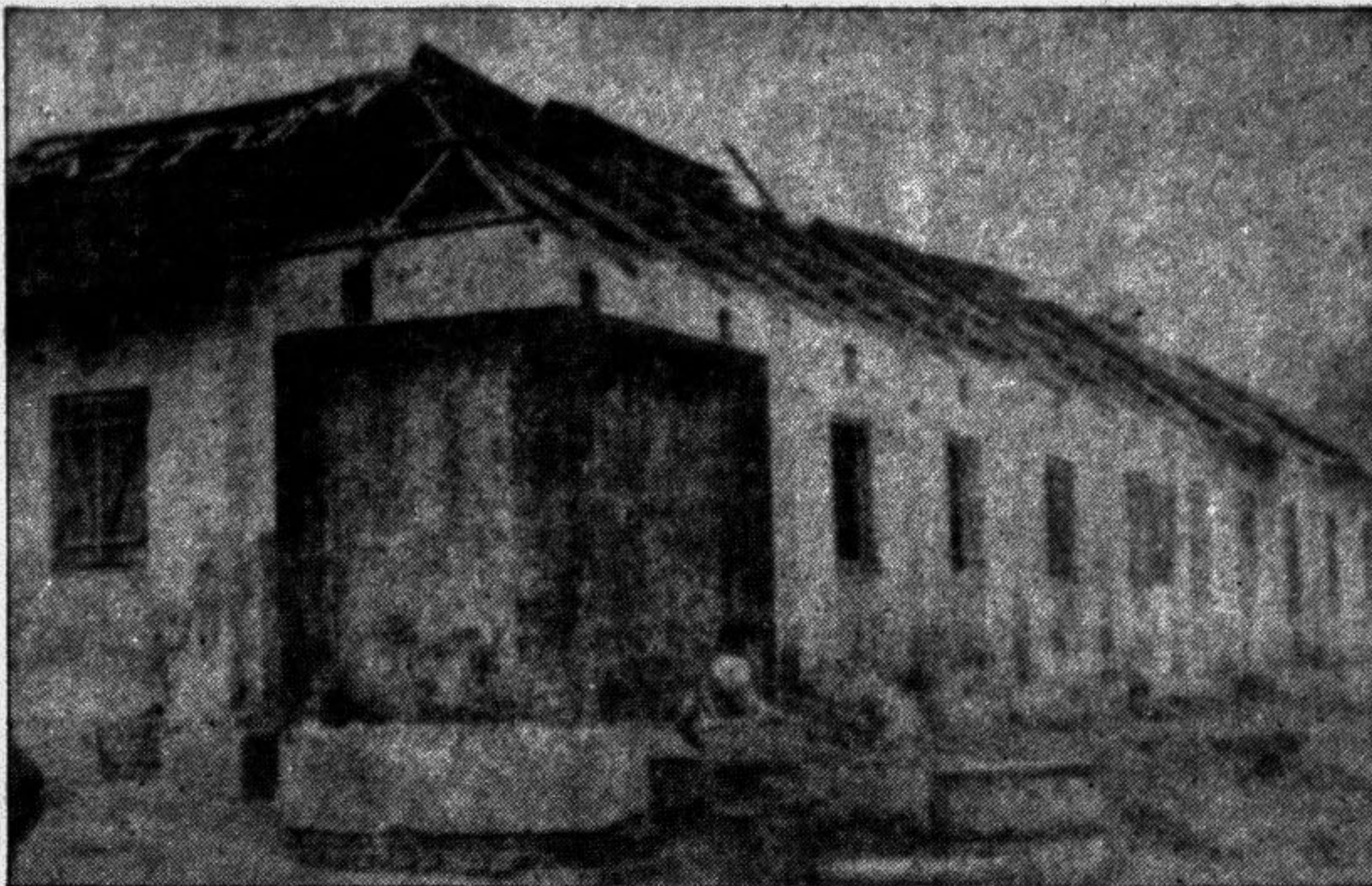
RANGPUR: Local Jummapara Government Primary School has not yet been repaired which was damaged by a cyclonic storm recently. — Star photo
