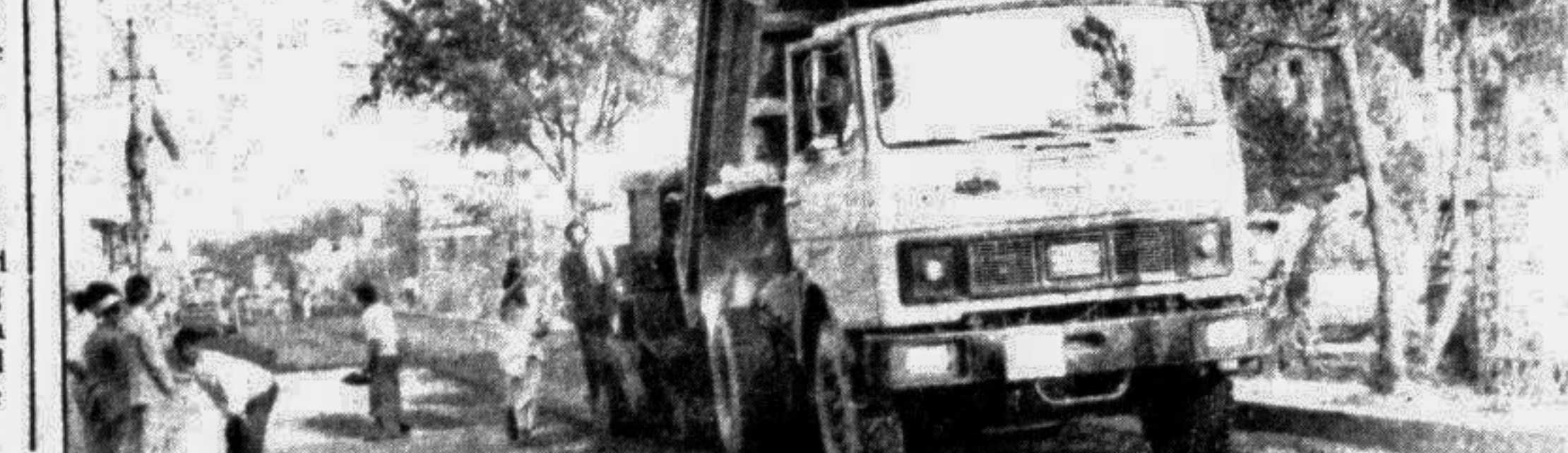
A DCC WHIM SENDING PEOPLE TO SPIN: A during-the-day repair work closed the road from Shahbag to Kataban intersection Thursday triggering off traffic jam in different parts of the city much to the disadvantage of the commuters in the peak hours. — Star photo
