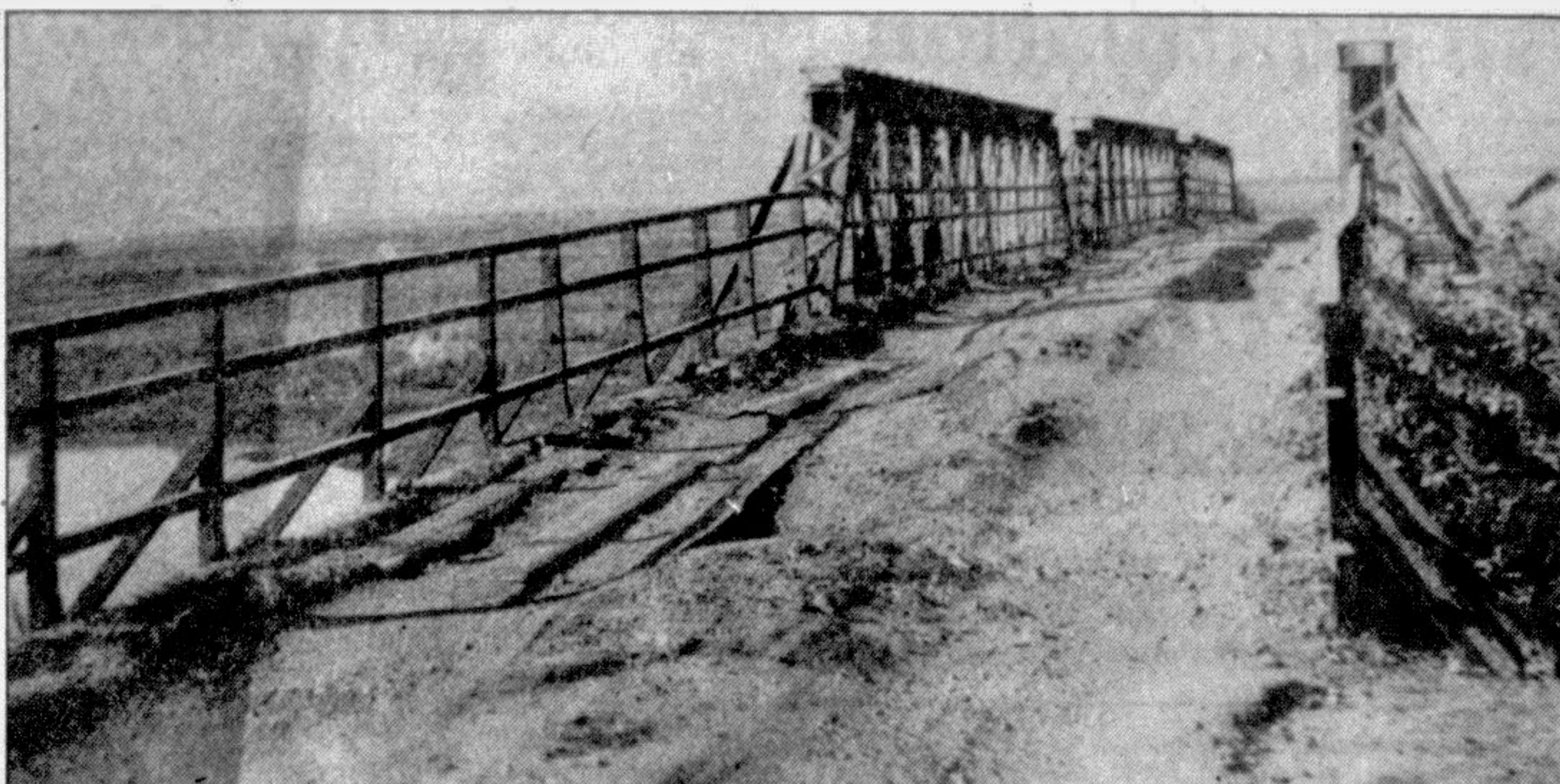
SYLHET: Dilapidated condition of a bridge on the Sylhet-Salutikor road which needs immediate reconstruction.
