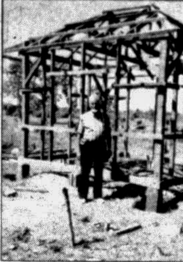
Completed Core Shelter Unit Frame during training at Lucena City (left) and houses occupied by inmates after completion (right).
